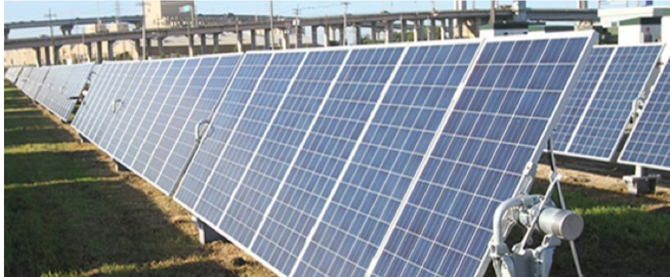
Entergy New Orleans' utility-scale solar plant is one of only a few in the U.S. to integrate state-of-the-art battery-storage technology.
