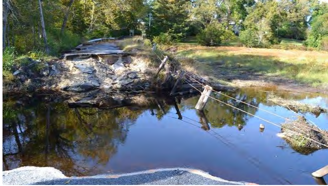
Photo 2. The dam and road at Barren Creek Pond failed during a severe July 2016 storm. The County rebuilt the roadway but did not restore the dam. Photo by Liz Holland.
