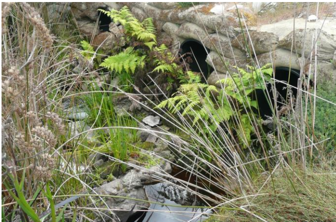
Photograph 4 - Shows the existing water crossing on the nearby Summertime Track. The crossing shows multiple culverts with concrete filled sandbags as scour protection.
