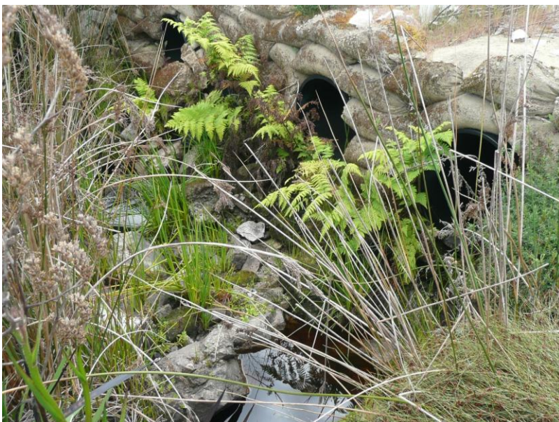
Photograph 9 here shows the existing water crossing on the nearby Summertime Track. The crossing shows multiple culverts with concrete filled sandbags as scour protection.
