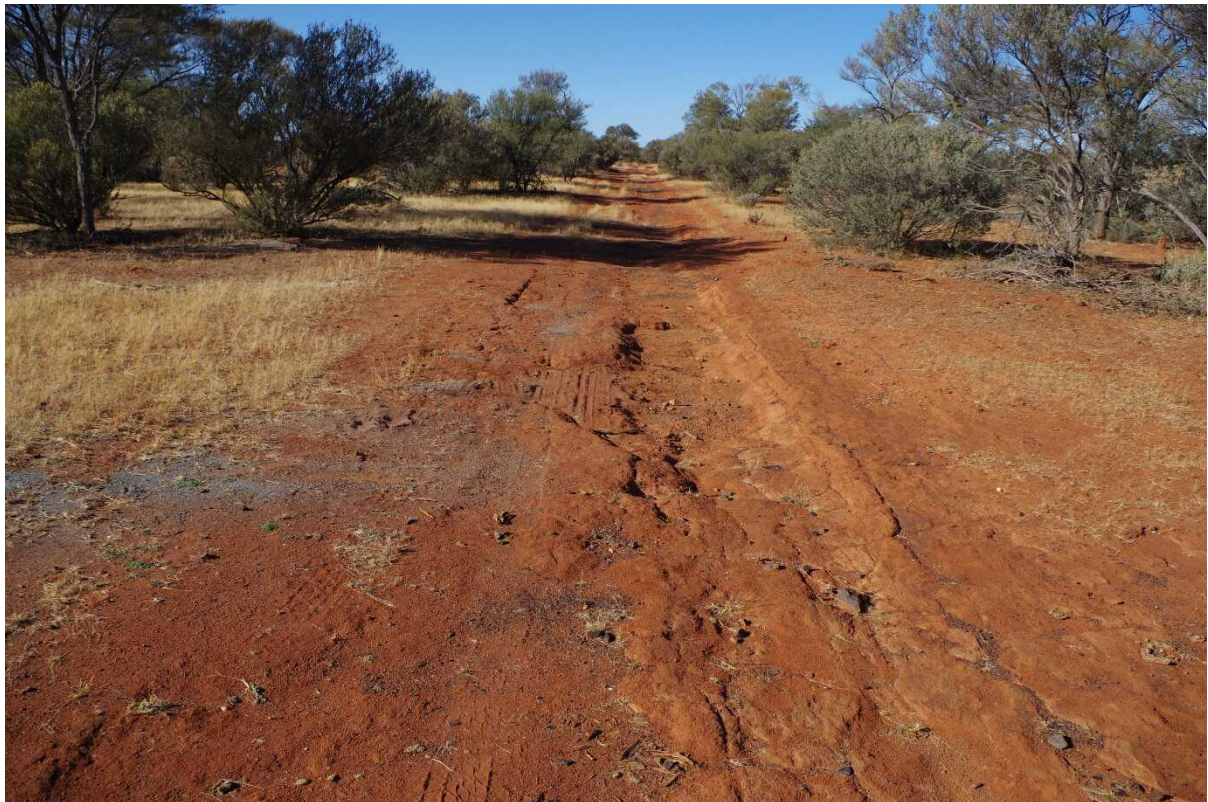
Photo 4 Scour resulting from flow concentration along a track near the south site
