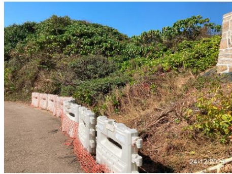
Collapsed fencing to be rectified
