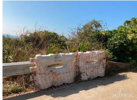
Collapsed fencing to be rectified
