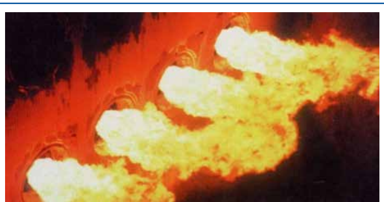
Pulverised fuel (PF) boiler showing four burners in operation during plant start-up
