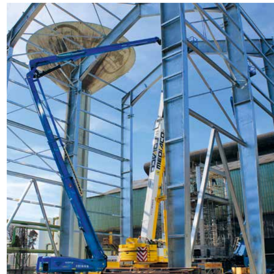
Construction of a new building housing Valdi's battery and catalyst recycling activity in Commentry (France).
