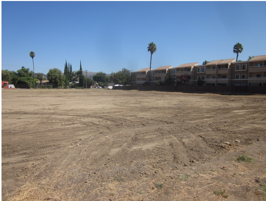
Overview of graded/excavated dirt in western portion of APE (view to NE)
