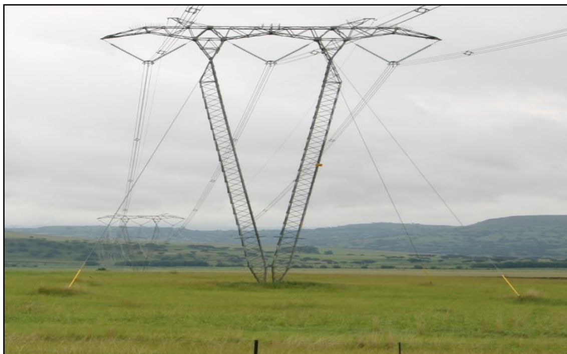
Figure 5: Guyed-V Suspension tower
