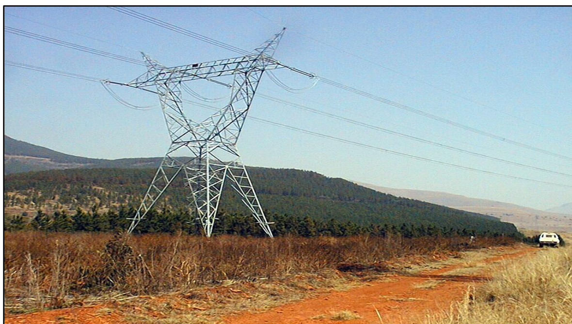
Figure 6: Self-supporting suspension tower
