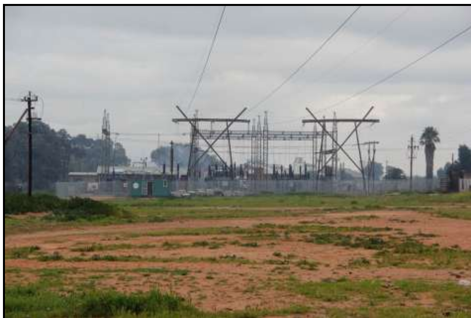
Figure 30. An area that would have originally been Grootkop Apronveld around the Oudtshoorn Substation, now completely disturbed and transformed.
