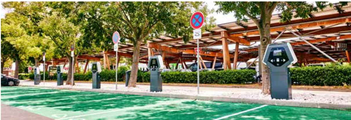
Electric car charging stations at Centr'Azur
