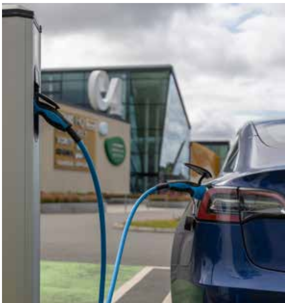
Charging station C4
