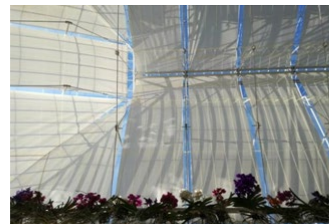
Figure 5: Automated ceiling screens
