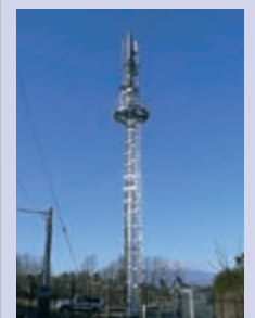
Mobile phone base station
