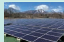
Mega solar power plant
