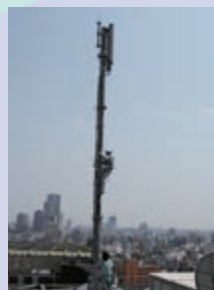
Mobile phone base station
