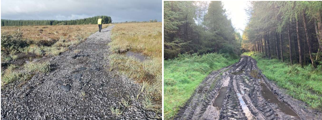
Figure 78 Existing trail in poor condition on the Lung Lough Gara Way
