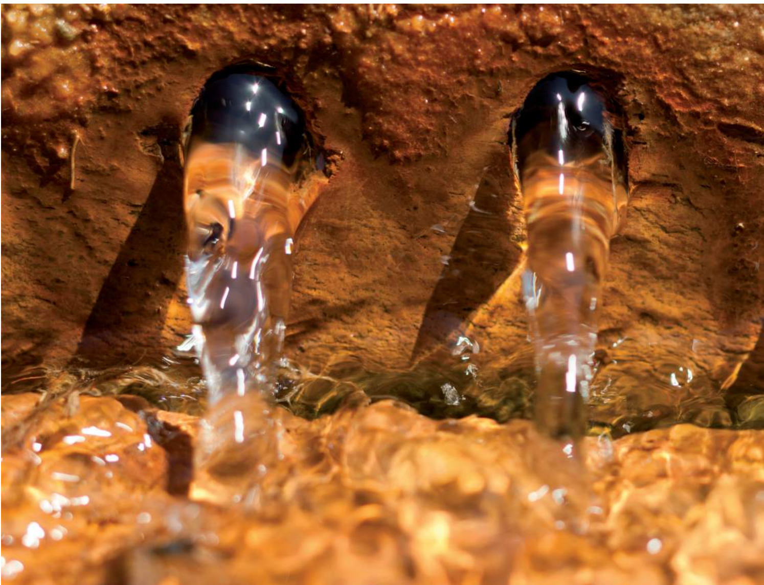
Salt water flowing from the main distribution junction.
