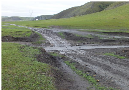
(a) Road Conditions Deteriorated by Runoffs
