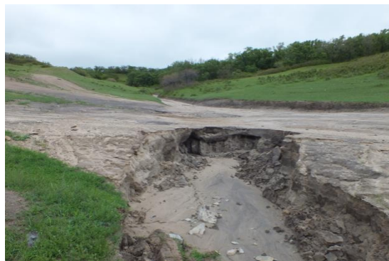
(b) Road Threatened by Erosion Gully
