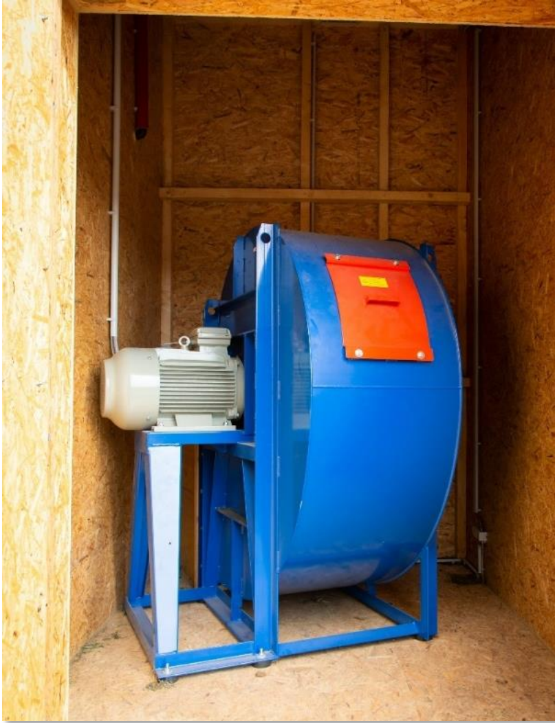
Figure 56 A ventilator blows (warm) air into the hay.
