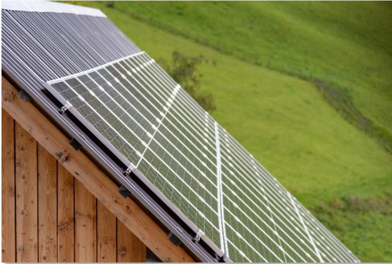
Figure 60 The energy required for hay drying is often covered by photovoltaics.
