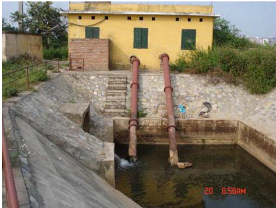
Figure 15: One of the electrically powered wastewater pumping stations for Bang B village from the Tor Lich River. Photo courtesy of William Leschen.
