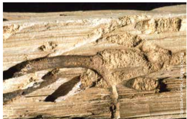
Damage (pupal galleries) caused by Giant wood wasp
