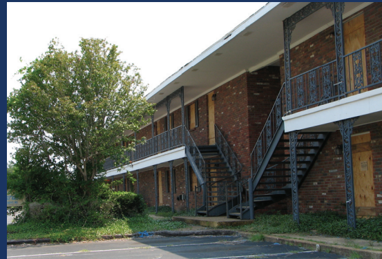
Exhibit 1-4: Damaged Rental Units
