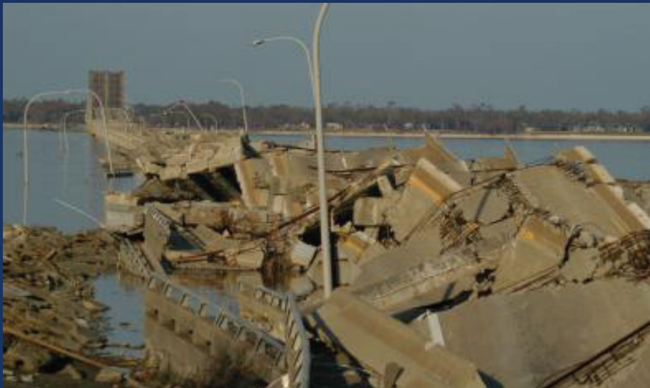
Damage to the Highway 90 bridge from Biloxi to Ocean Springs.
