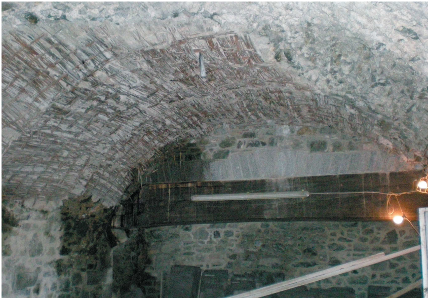
Plate 31 View of reconstructed stone vaulted ground floor with wicker centring and timber lintel to open range fireplace in background
