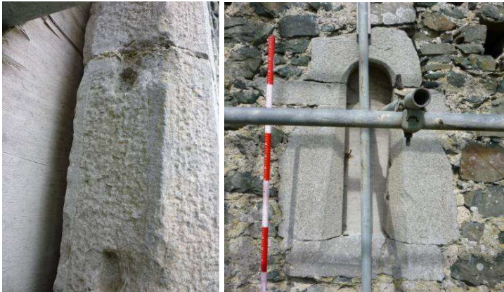
Plate 43 Original window detail. The original round headed loop window (at the southern elevation) has splayed jambs flared toward the base. Some of the new openings replicate this style. To the upper right of the loop is a possible putlog hole.
