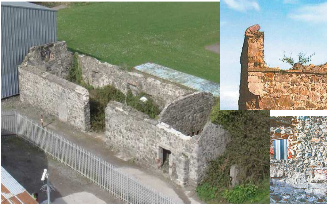
Plate 37 Aerial view of the outbuilding, view of the the northern gable and damaged window ope
