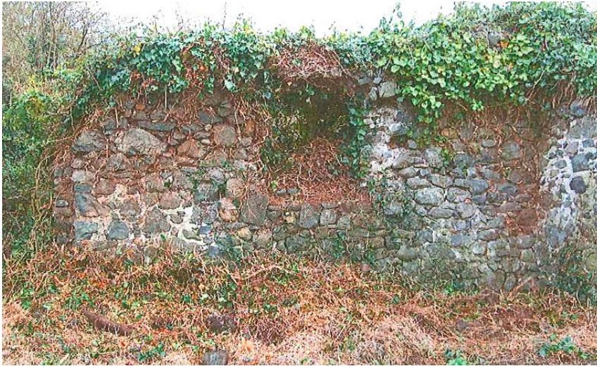
Plate 38 St Molaga's Church - masonry has been engulfed and eroded by vegetation
