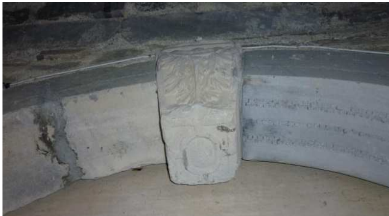
Plate 12 Architrave now inserted into the internal porch at the principal seventeenth century entrance into the monument
