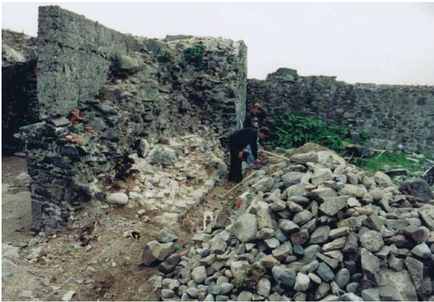
Plate 21 View looking south along the southwestern wall, indicating what little had survived of this elevation. At this location the wall had been broken through in antiquity, a new doorway and porch has been constructed and a new stone spiral stair well
