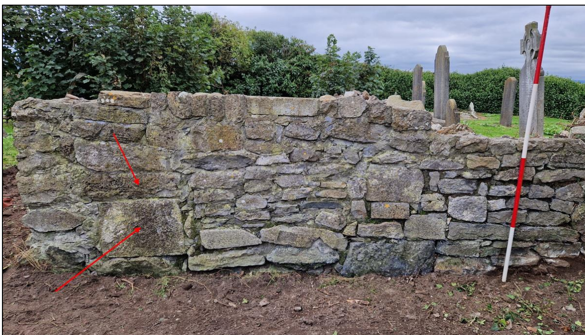
Plate 12 Interior south wall, previous reconstruction work west of entrance. Reused architectural stone indicated
