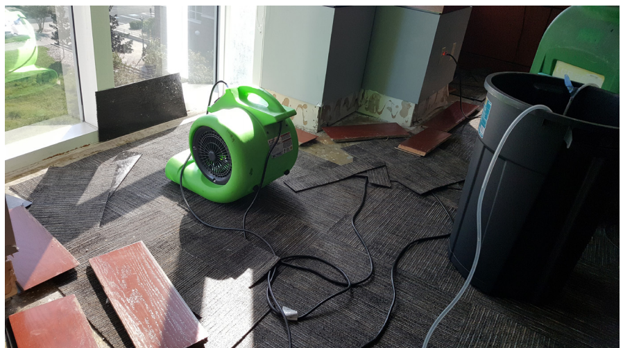
Vast portions of Florida suffered flooding from Hurricane Irma, which made landfall in the Florida Keys in September 2017. The biggest problem for many of the state’s courthouses was water damage, as was the case for this courtroom in the Charlotte County Justice Center.
