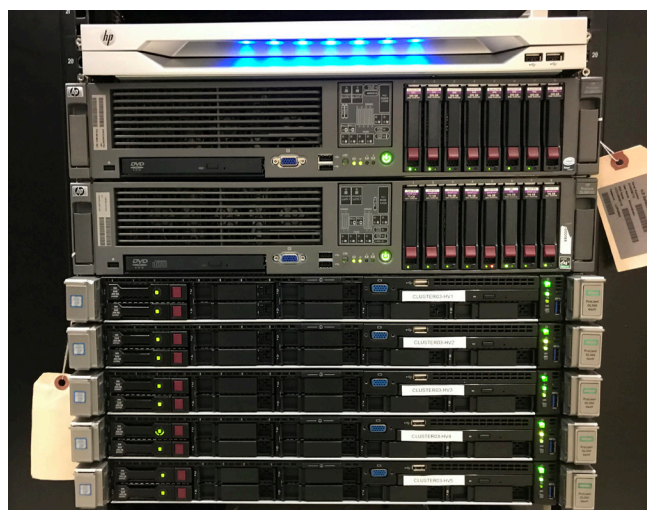
The five new Generation 9 servers (pictured in the bottom half of the photo) will replace more than 60 of the old Generation 6 servers (two of which are pictured at the top of the photo).
