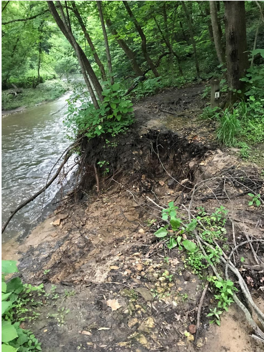
Trail damage by Franklin Creek
