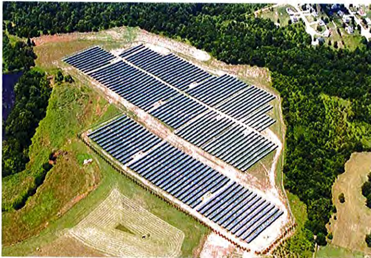
Figure 1: Utility-scale solar facility (5 MW DC ) located in Catawba County. Source: Strata Solar
