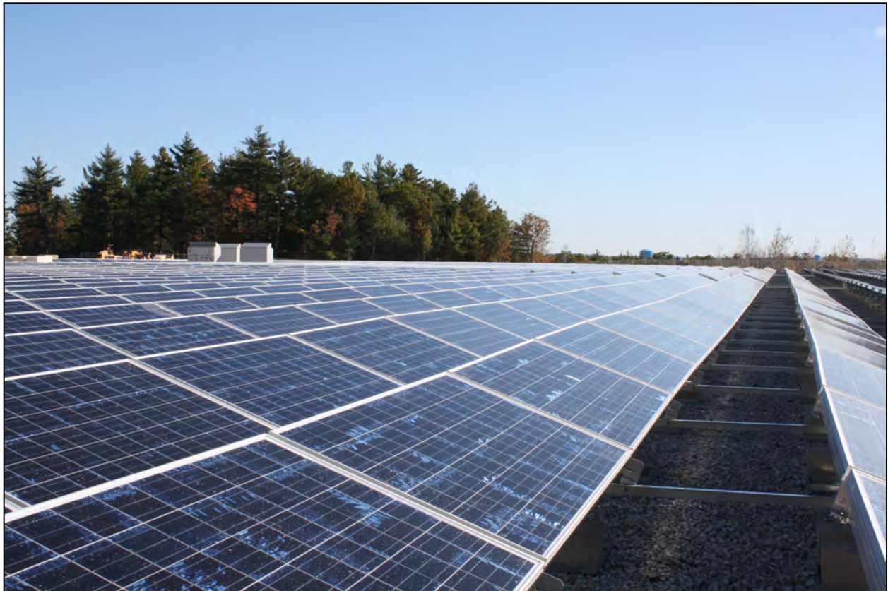
Westford Solar Park, photo courtesy of EEA
