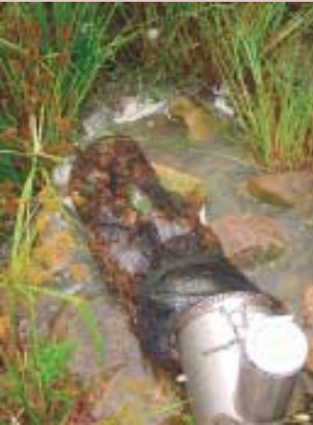
Nettech device off Clarinda Street, Hornsby
