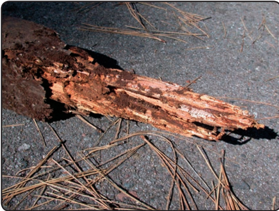
Figure 173. Damage to sign post caused by termites.
