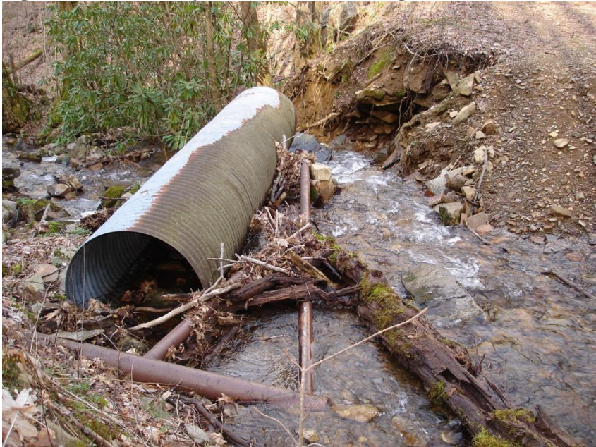
Figure 3.3.1. Hickory Cove Creek crossing blow-out.
