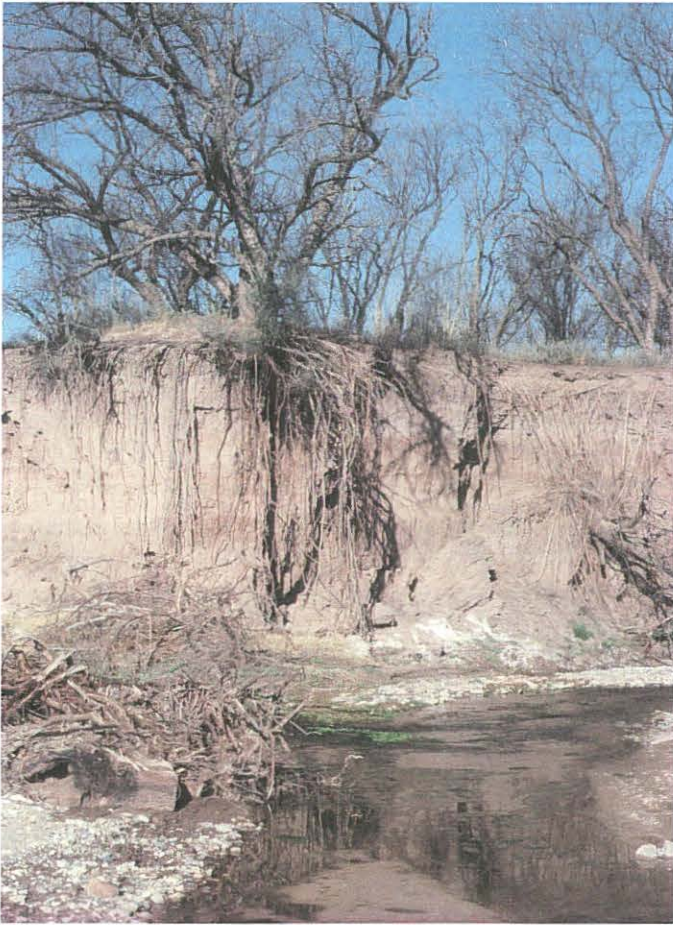
Figure 7. Eroded bank along Cienega Creek, Arizona, 1977. Mesquite, growing on the elevated terrace, forms deep roots in pursuit of a declining water table, quickly replacing cottonwood-willow riparian woodlands after channel incision.
