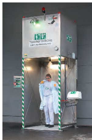
Tanknotduschen Tank safety showers
