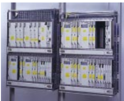
Fujitsu Laboratories and Fujitsu Limited have developed a WDM system, shown here, that processes a 10-gigabit optical system in 32 wavelengths. Other noteworthy R&D advances include successful prototypes of an Optical Add/Drop Multiplexer (OADM) and an Optical Cross-connect System (OCS).
