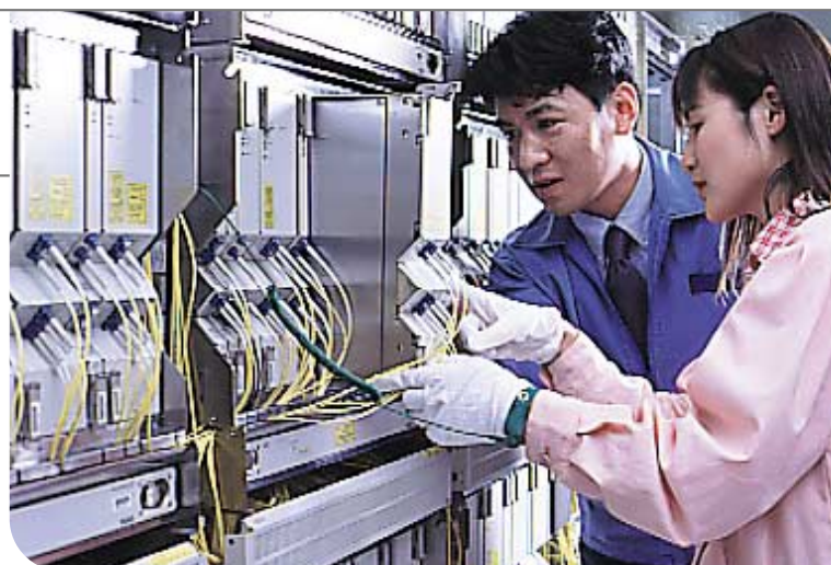
Testing of WDM system equipment
