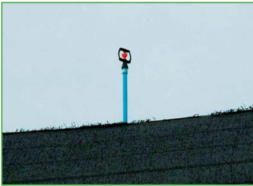
Figure 12. Sprinkler on the roof (Photo courtesy of Tawat Tapingkae)
