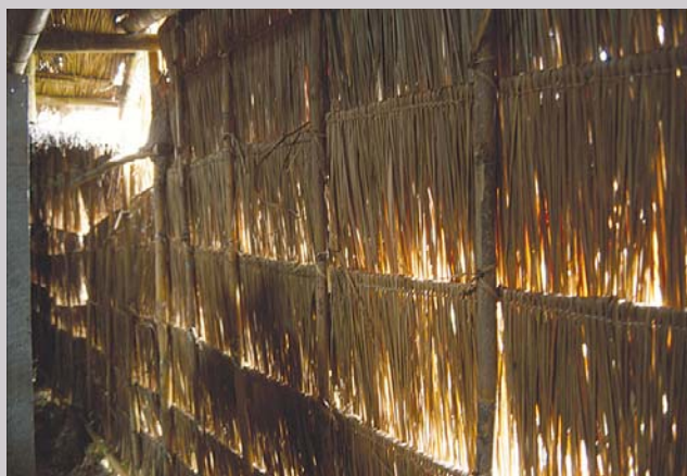
Figure 15. Light leaking into growing house
