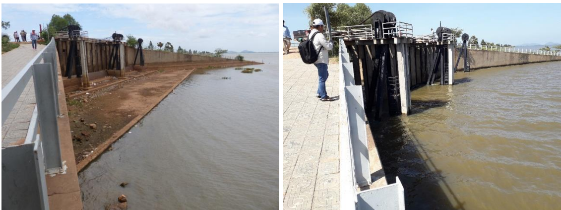
Photos 6a & 6b: ATT sluice gates on 1 st July 2019 (left) and 18 th October 2019 (right)
