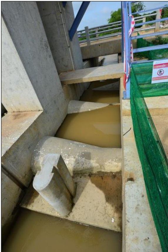
Photo 1: Looking down Wat Chre fish-pass Headwater levels are too low so there is no flow through it. Note the unused slots for gates which could control inflows.
