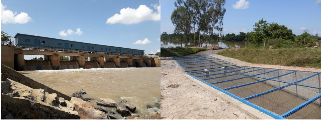
Photos 27a & 27b: Damnach Ampil headworks (left); wire mesh covered fish pass (right), upper inlet section.
