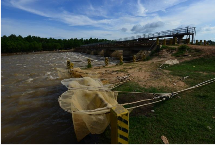
Photo 18: Charec Weir, Pursat River, moderate discharge on 8-10-19 There is no fish pass at this site. Fish passage is inhibited by strong turbulence and fast flow, despite relatively little drop across the gates. Note the fishing nets used by people targeting fish which are obstructed at the barrier.
