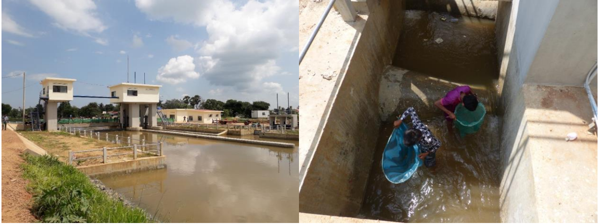
Photos 24a & 24b: Ream Kon headworks, with irrigation canal intake to the right (left); boys with dipnets in the fish pass (right)
