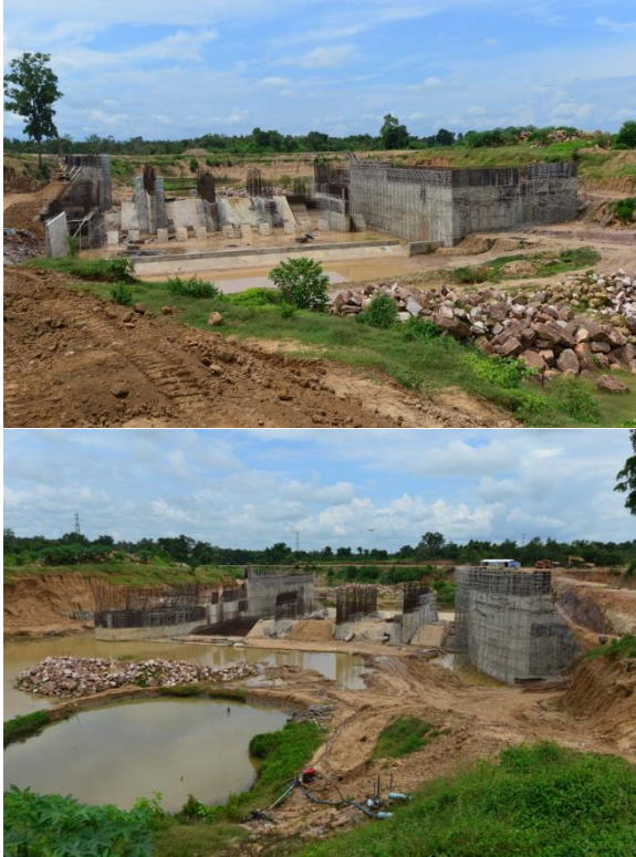
Photos 11a & 11b: Damnak Choeur Krom dam site looking upstream (left) and downstream (right)
