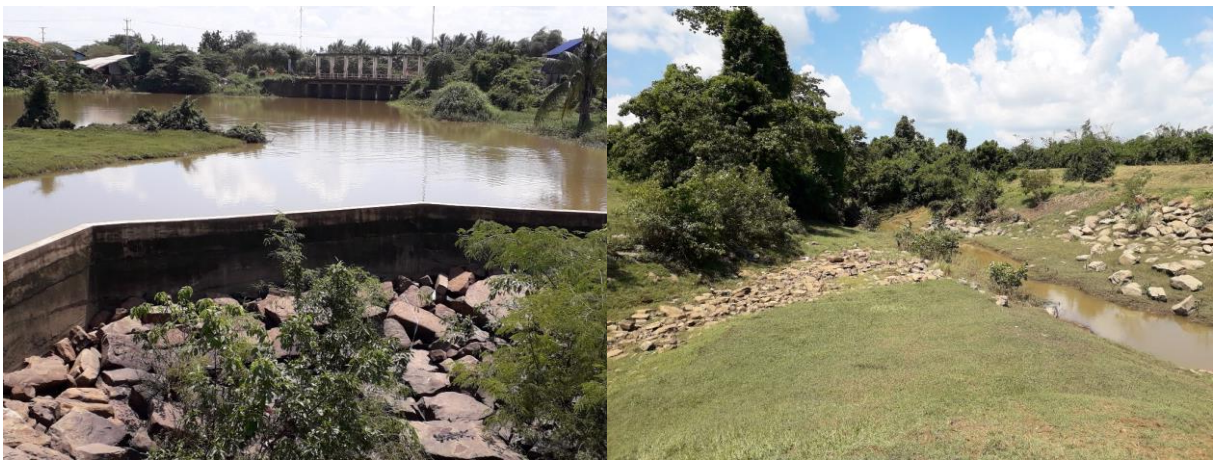
Photos 23a & 23b: Spillway of Prek Chik dam (foreground) with intake for primary irrigation canal in background (left); only standing water in the Stung Moug Russei river downstream of the Prek Chik dam (right).
