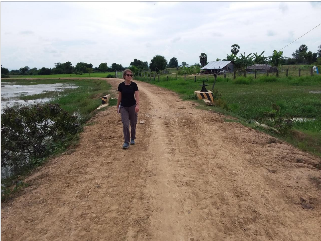
Photo 34: Ang Beng CFR, showing road which cut flows, and culvert which was later installed
