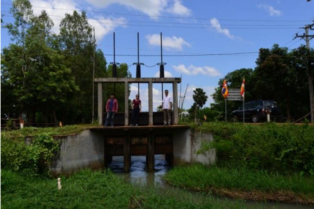
Photo 21: A typical top-down water-gate to irrigation canal from Tang Krasaing Reservoir While fully open fish can pass, but when partly closed fish may be injured or killed by passage
