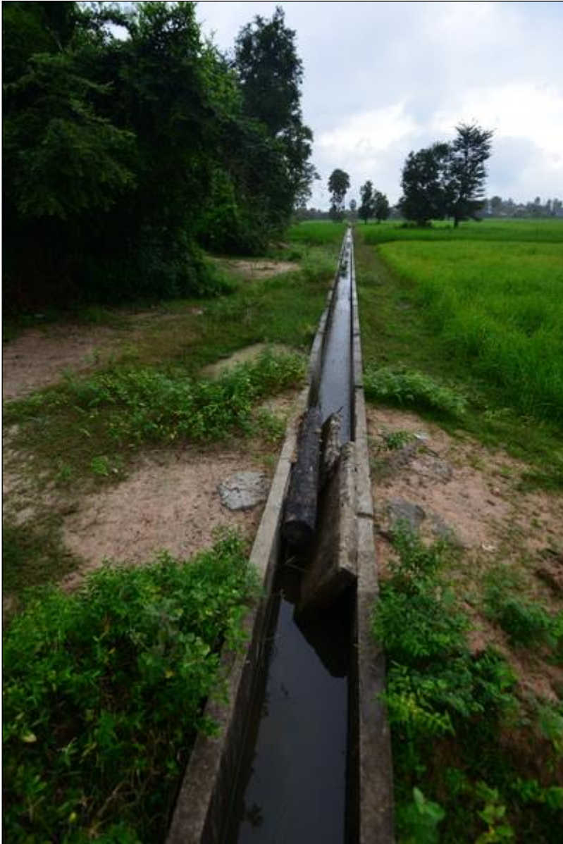
Photo 32: Boeng Kantout CFR concrete irrigation canal which cut off the flow to the CFR The CFR members had to install culverts to provide flow under the canal, which is apparently not used.
