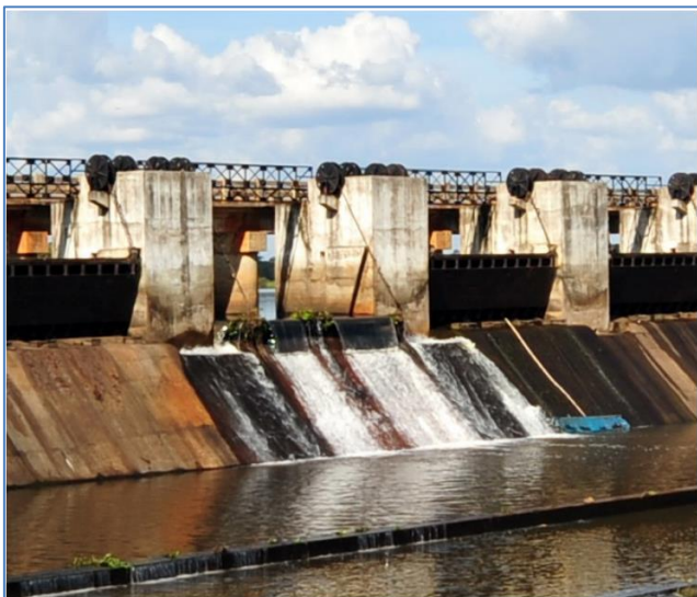
Figure 21: Overshot water-gates on Tumhub Makak Dam, Kampong Thom, Cambodia
