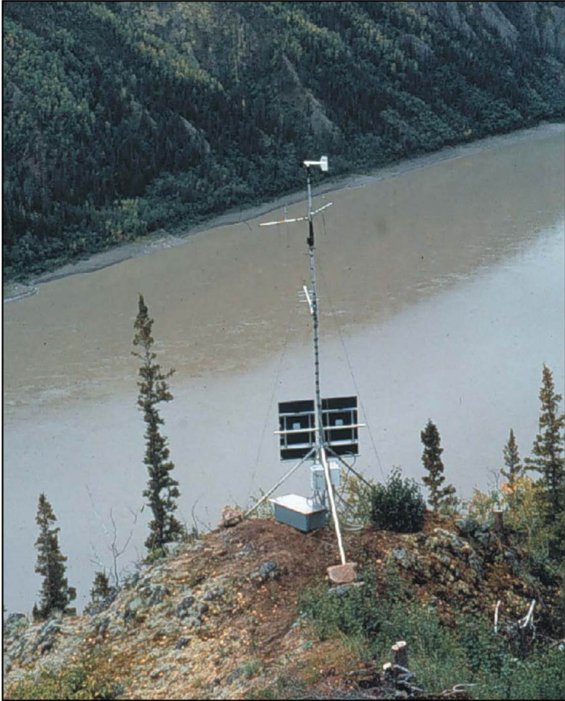
Figure 27. A remote, radio receiving station located high on a bluff along the Yukon River. Solar panels (dark rectangles low on the tower) charge the batteries that power the receiver. Antennas mounted high on the tower point upstream and downstream, allowing the passage direction of radio-tagged fish to be determined based on the strength of the radio signals. In recent years, numerous receiving stations such as this have been deployed around the Yukon and Kuskokwim River drainages to track fish migrations. Photo by J.H. Eiler, NMFS.
