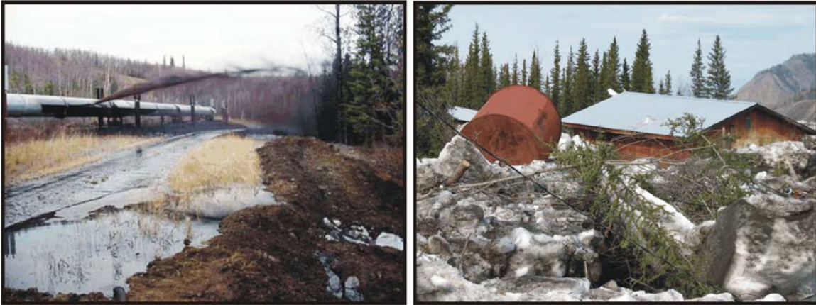
Figure 17. Images of the Trans-Alaska Pipeline shooting incident in October 2001 near Livengood, Alaska (left), and one of many dislodged and leaking fuel oil tanks in Eagle, Alaska following the extraordinary breakup of May 2009 (right). Photos courtesy of the Alaska Department of Environmental Conservation.
