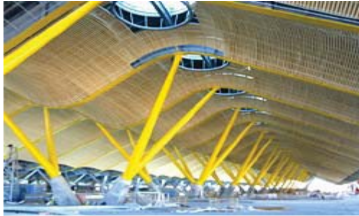
Bamboo lamination board used as fire-proof ceiling in Madrid airport, Spain
