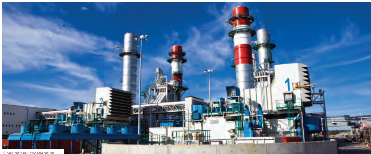
Sines refinery cogeneration
