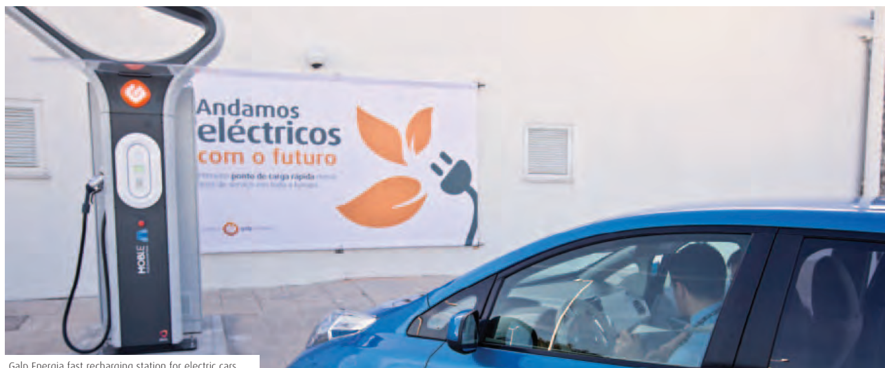
Galp Energia fast recharging station for electric cars
