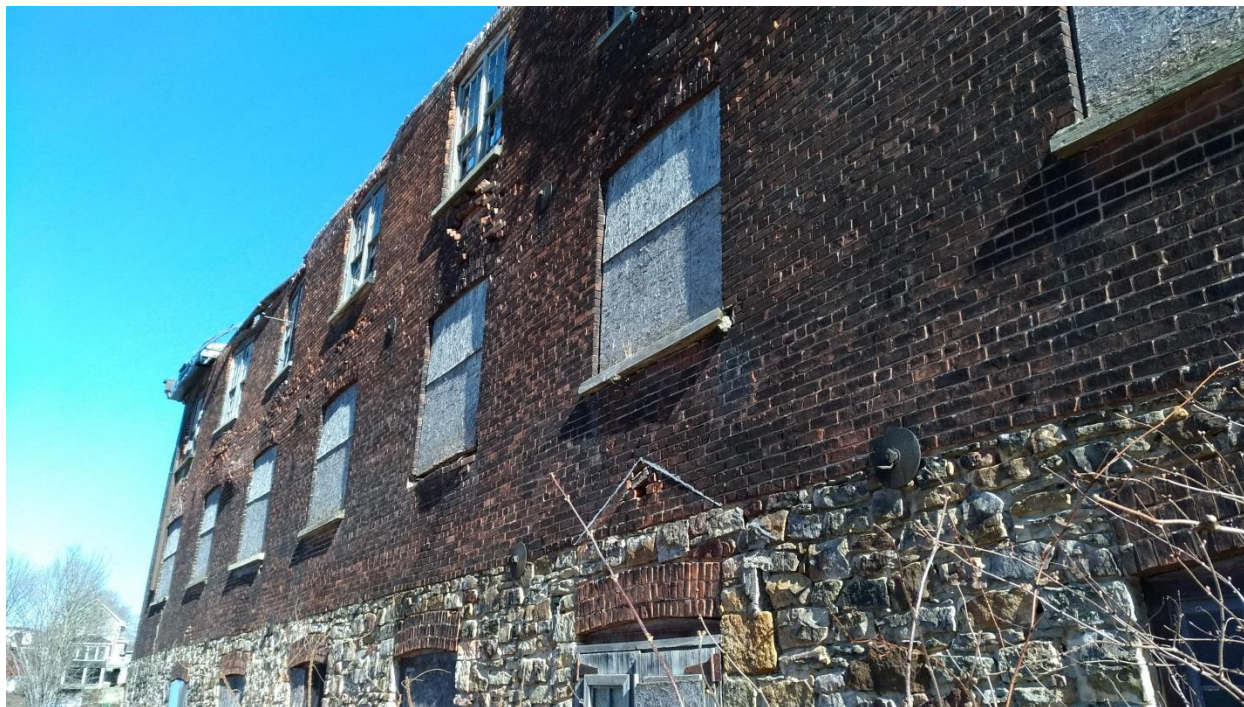
Figure 14: Brick Building, viewed from the northwest, showing the deterioration and bowing of the northeast wall (E. Tumak, March 2020).
