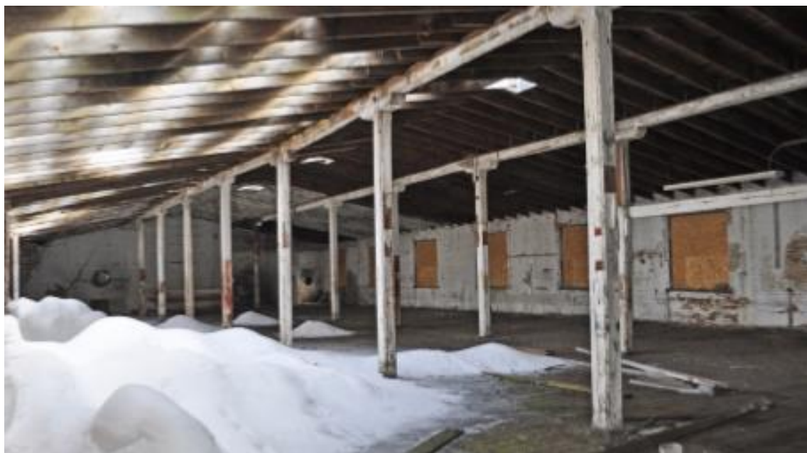
Figure 15: Brick Building upper level interior looking east, showing the breach in the roof at the northeast end as early as 2014, and the resulting moisture/snow infiltration (source, "185 Mill Street and 15 Clarence Street" Heritage Impact Statement, March 2014, Appendix A, p. 28).
