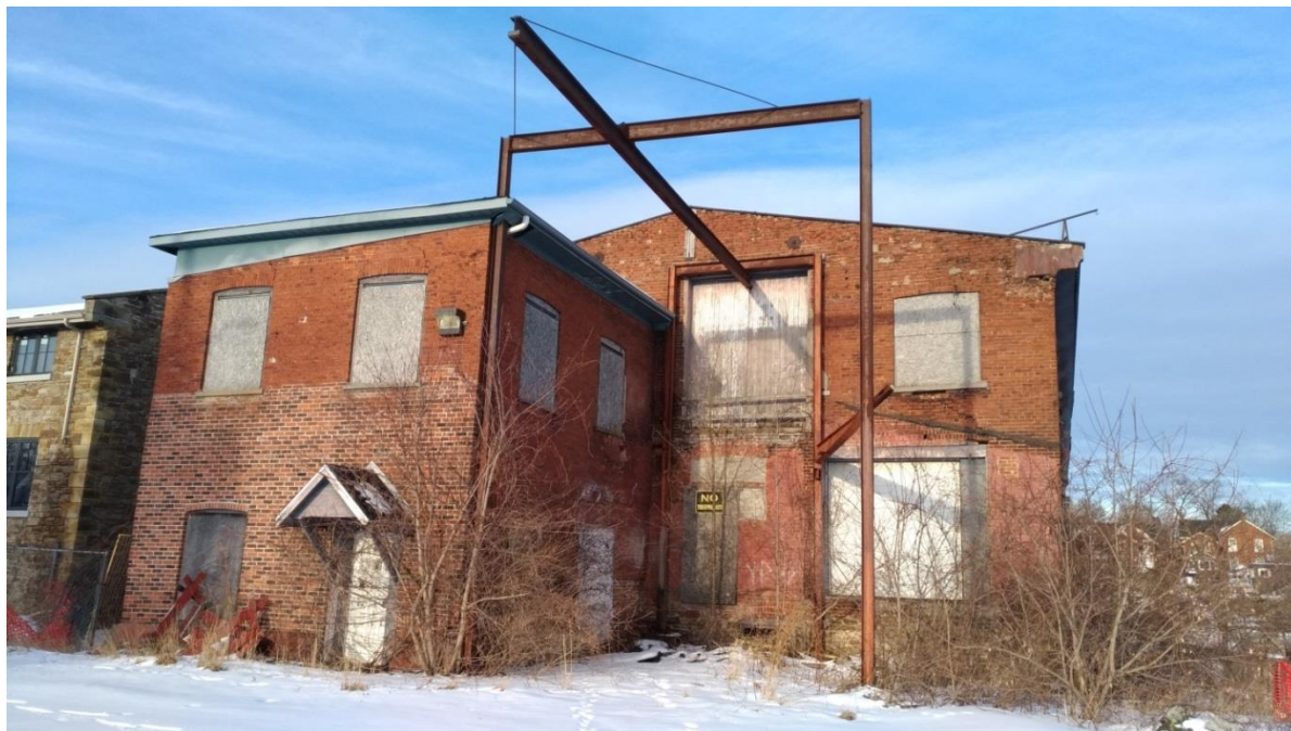
Figure 8: 185 Mill Street, Brick Building, west elevation. The two-storey brick extension in the foreground dates from ca. 1895-1900. (E. Tumak, Jan. 2020).
