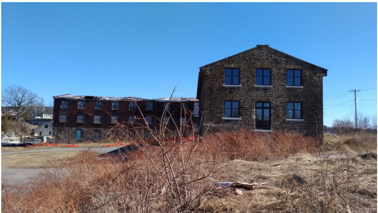
Figure 13: View from the north, showing the partially collapsed north roof of the Brick Building (E. Tumak, March 2020).
