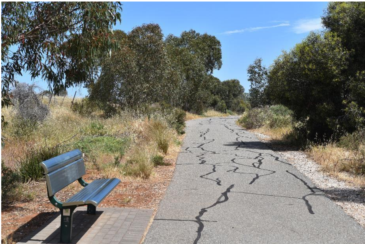
Below: A shared use track and rest stop with local native revegetation off Potts Road, Evanston Park.
