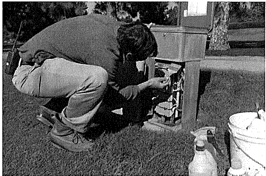
Clean field satellite controllers quarterly by dusting, removing cobwebs, and replacing insect repellent. This can greatly extend the life span of electrical components.
