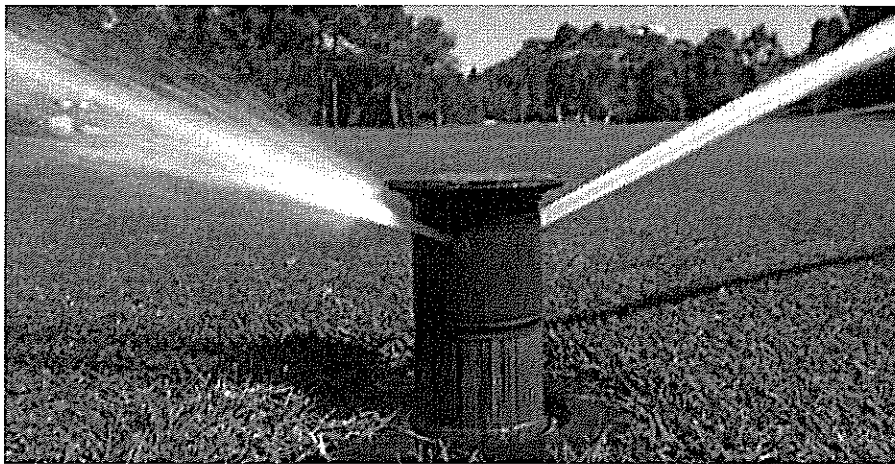
Sprinklers should be checked every week to ensure that they properly pop up, turn, and retract. Check that they rotate at the correct speed and that they are not leaking.
