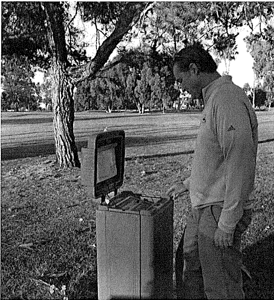
Checking the satellite controllers and central computer for backup programs and accurate run times should be done at least once every month.
