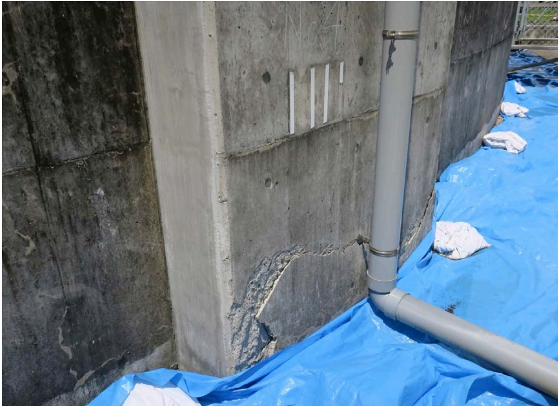
Figure 5-33. Damaged Tendon Anchor Point, with Incipient Spalling
