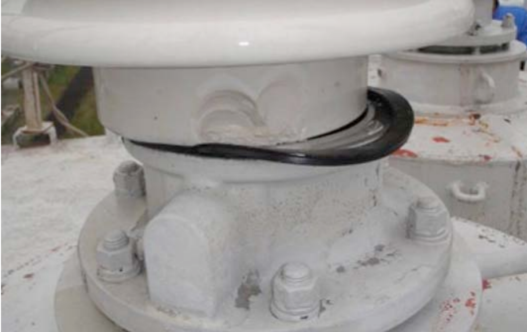
Figure 3-44. Damaged S Bushing for 66 kV Shunt Reactor in Figure 3-43
