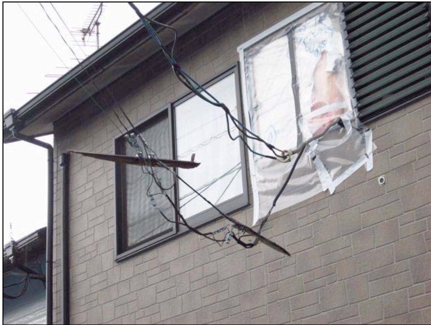
Figure 4-7. The drop wire connection was pulled from the exterior wall of this house in Mashiki town ( 32.7884^{\circ}\text{N} , 130.8184^{\circ}\text{E} ). Note the proximity of the power drop wire.
