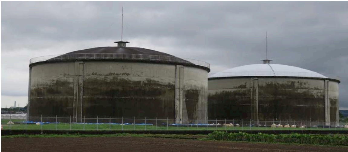
Figure 5-30. Two Pile-Supported Concrete Tanks
