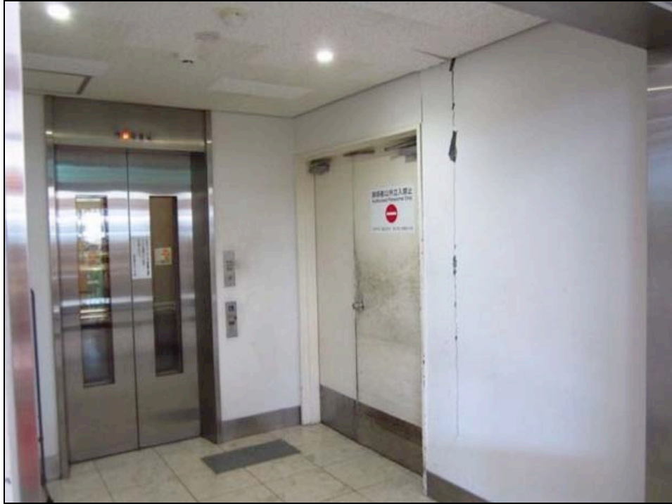
Figure 7-9. Cracks along the dry wall joints; the ceiling tiles were no damaged. The elevator was not damaged
