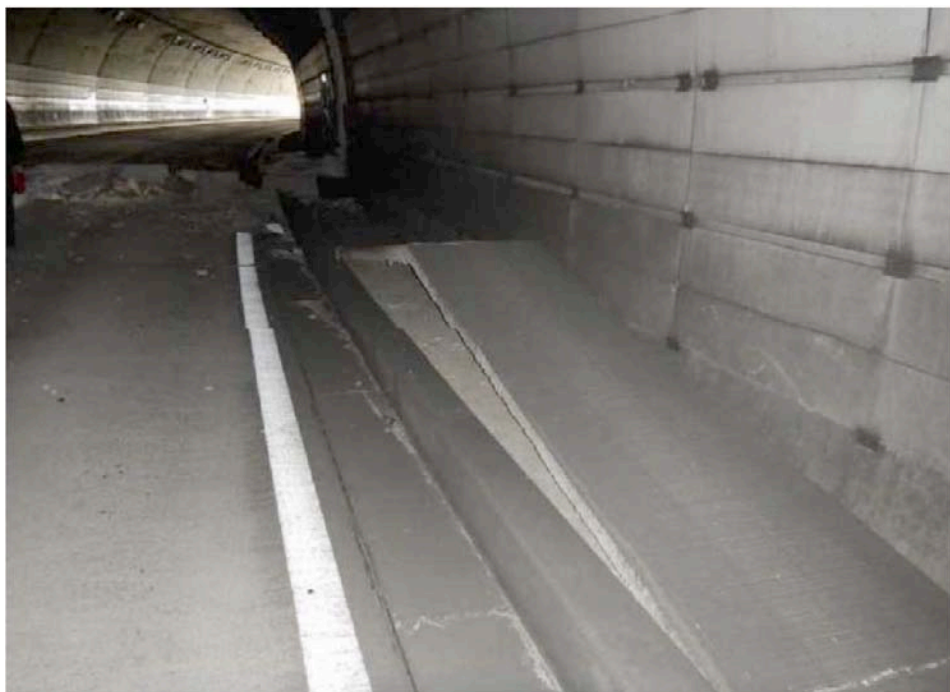
Figure 9-70. The side path concrete surface buckled
