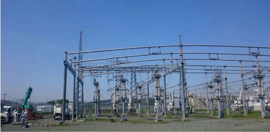
Figure 3-40. Damaged 220 kV Rigid Bus End Posts
