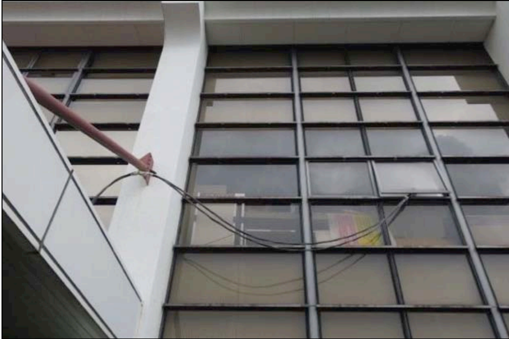
Figure 7-14. Two sets of telecommunication cables were installed to provide Internet service
