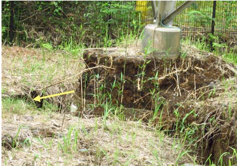
Figure 3-17. Old Tower 2 Ground Deformation
