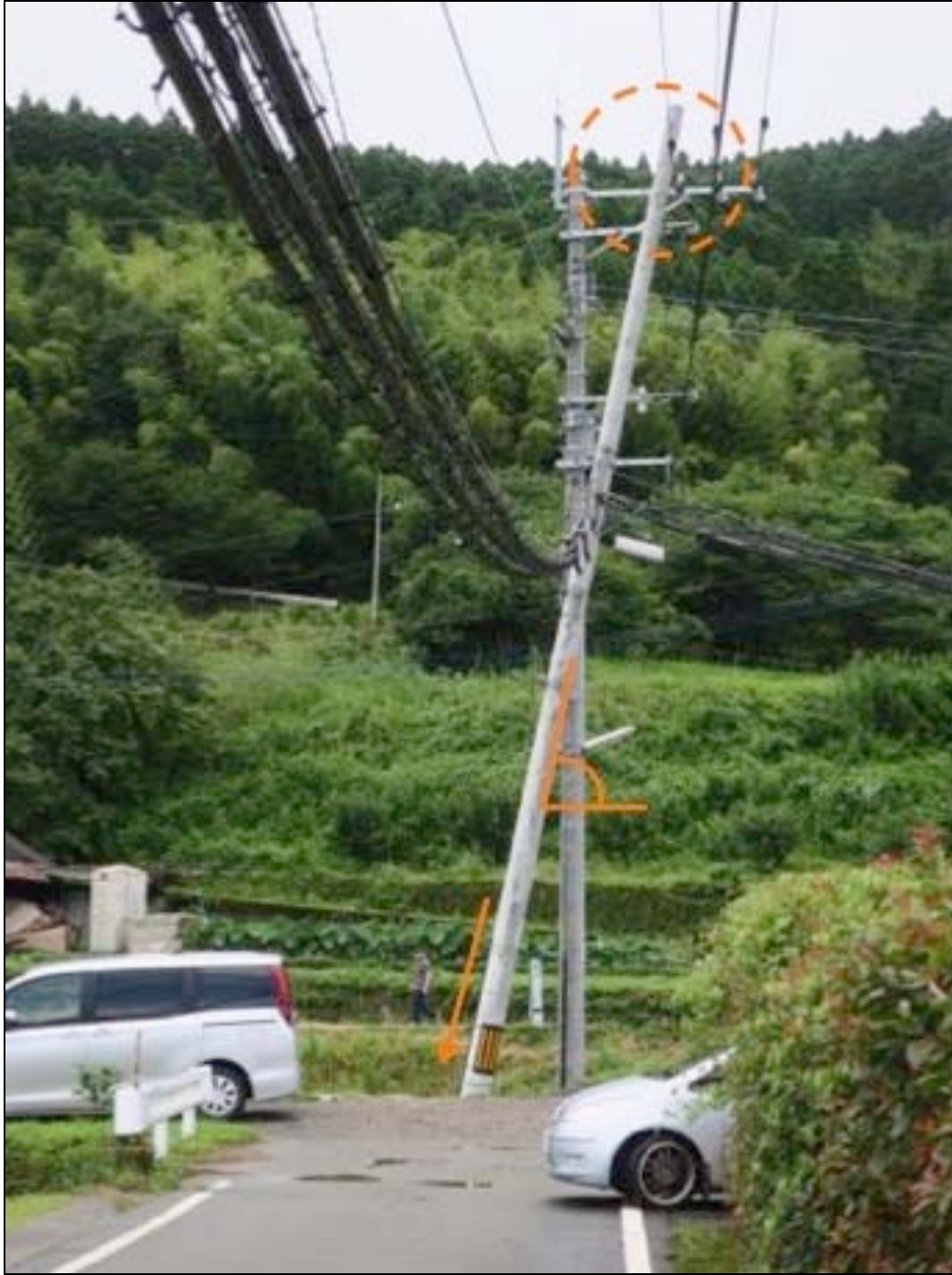
Figure 4-2. The utility pole carrying the telecom aerial cable bundles sustained ground failure damage. The top part of the pole was resting on the power cable isolator
