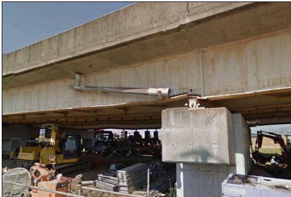
Figure 9-21. Broken drain pipe due to bridge movement
