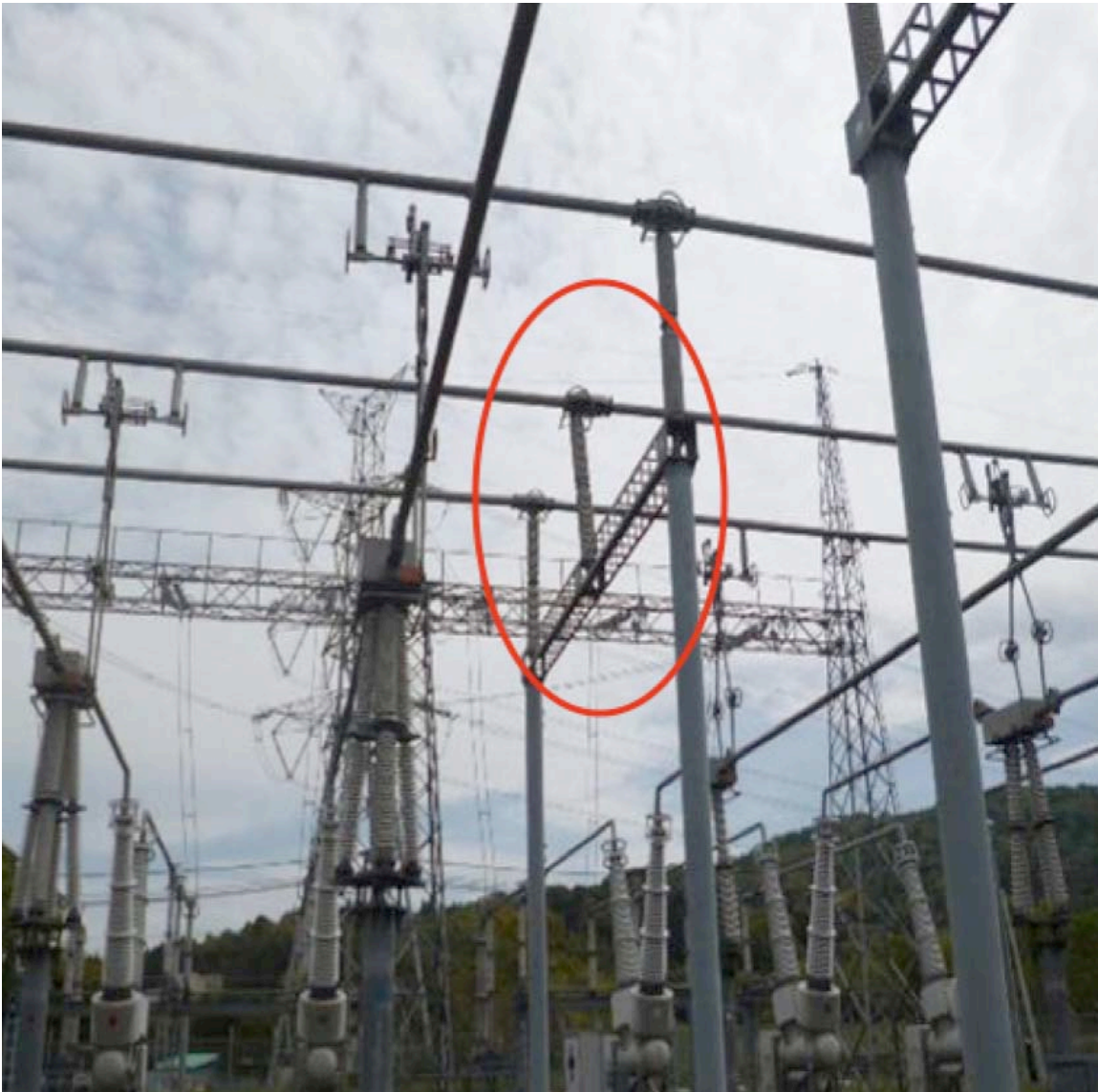
Figure 3-41. Damaged 220 kV Rigid Bus Post
