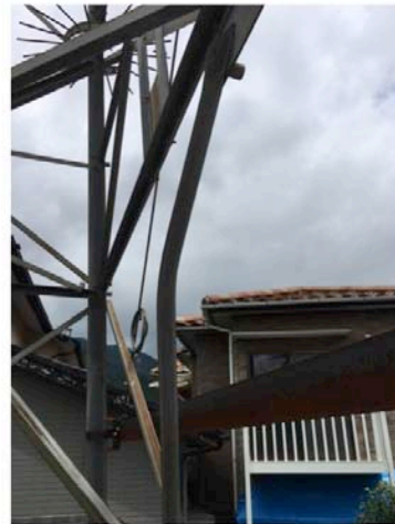
Steel Tower 10 Buckled Brace
