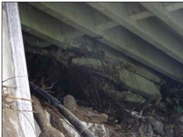
Figure 9-55. This is under the deck just before the landslide that destroyed 30 m of the bridge
