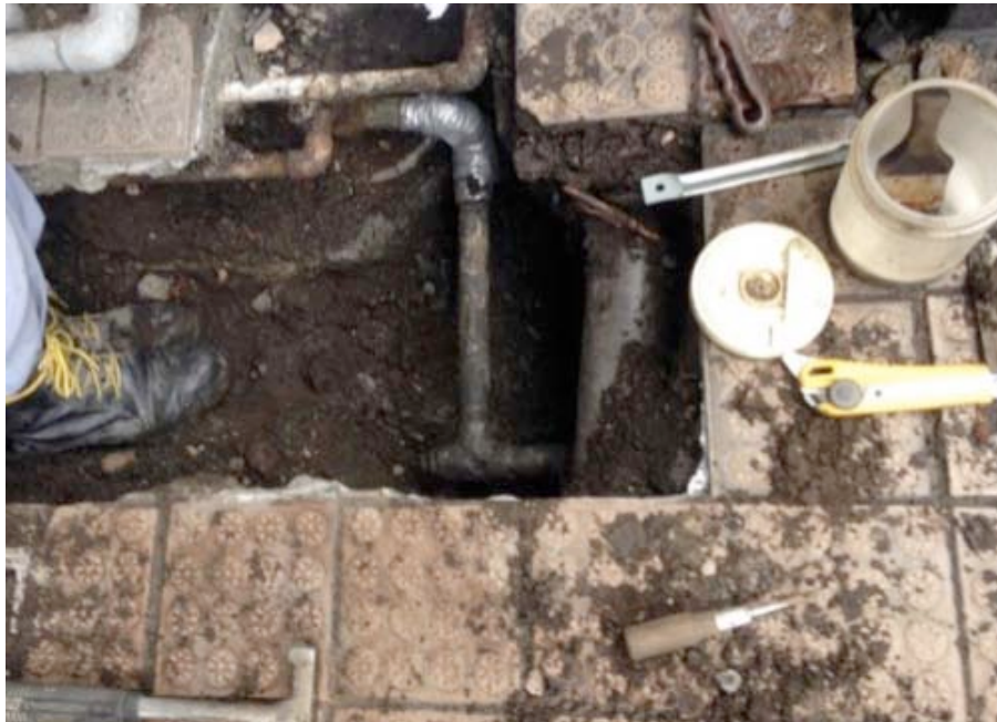
Figure 8-13. Damaged Low Pressure Pipe Customer Service Lateral
