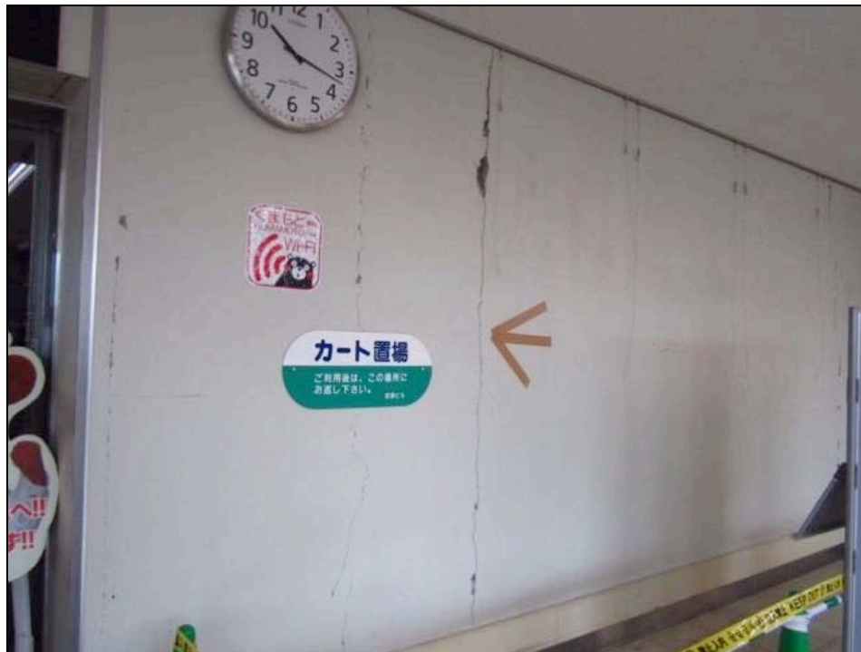
Figure 7-8. Cracked dry wall joints in the waiting area
