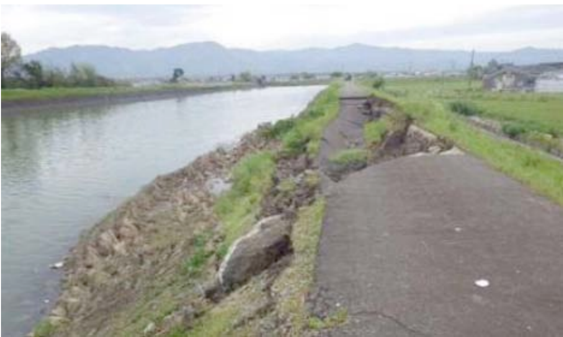
Figure 10-3. Levee Damage. Oosakawa River (Yatsushiro River). Masonry seawall collapse
