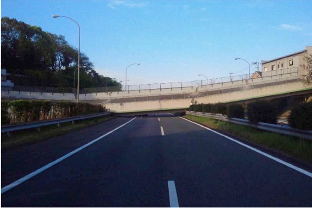
Figure 9-24. The collapsed bridge blocked the northbound traffic
