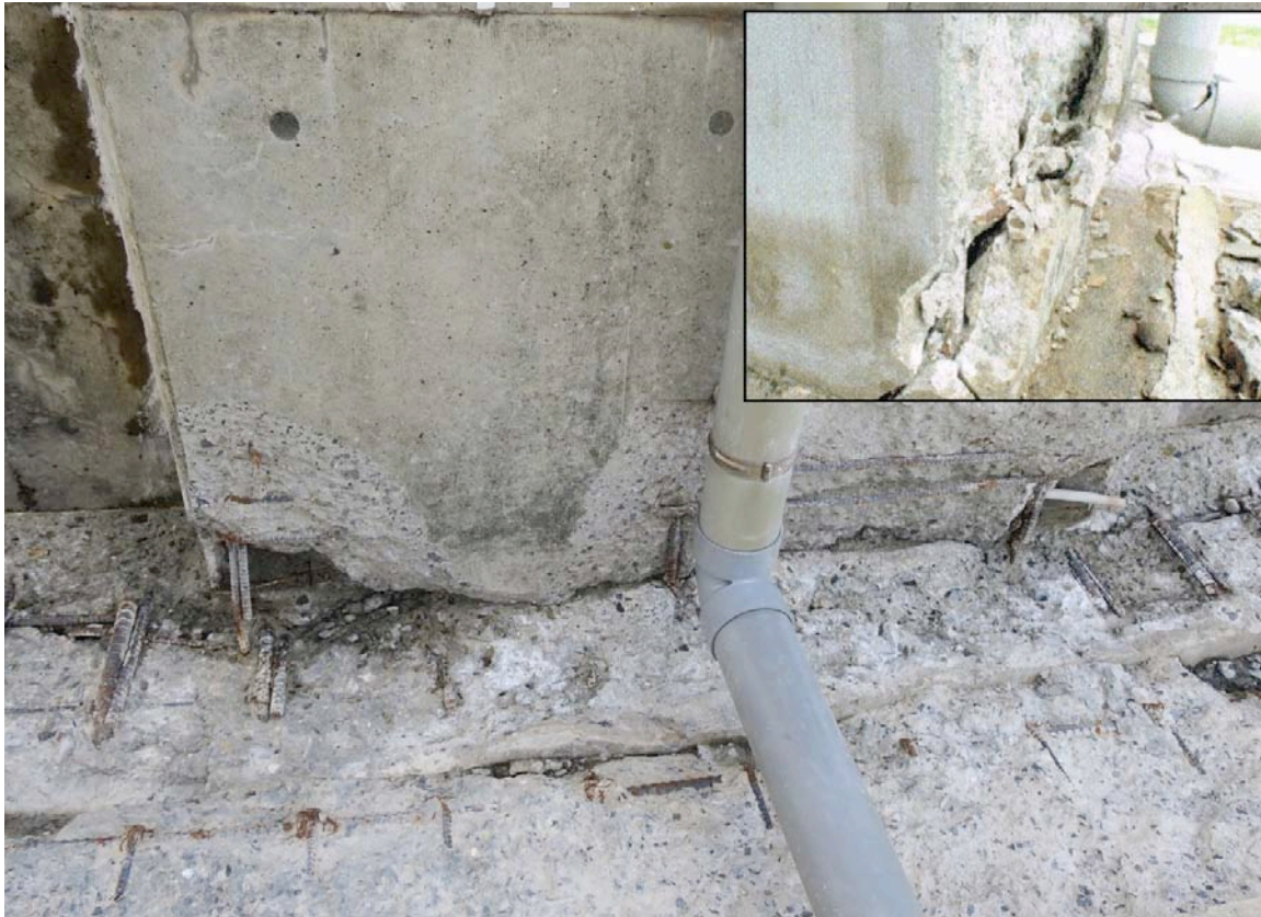
Figure 5-32. Damaged Tendon Anchor Point, with Gross Spalling
