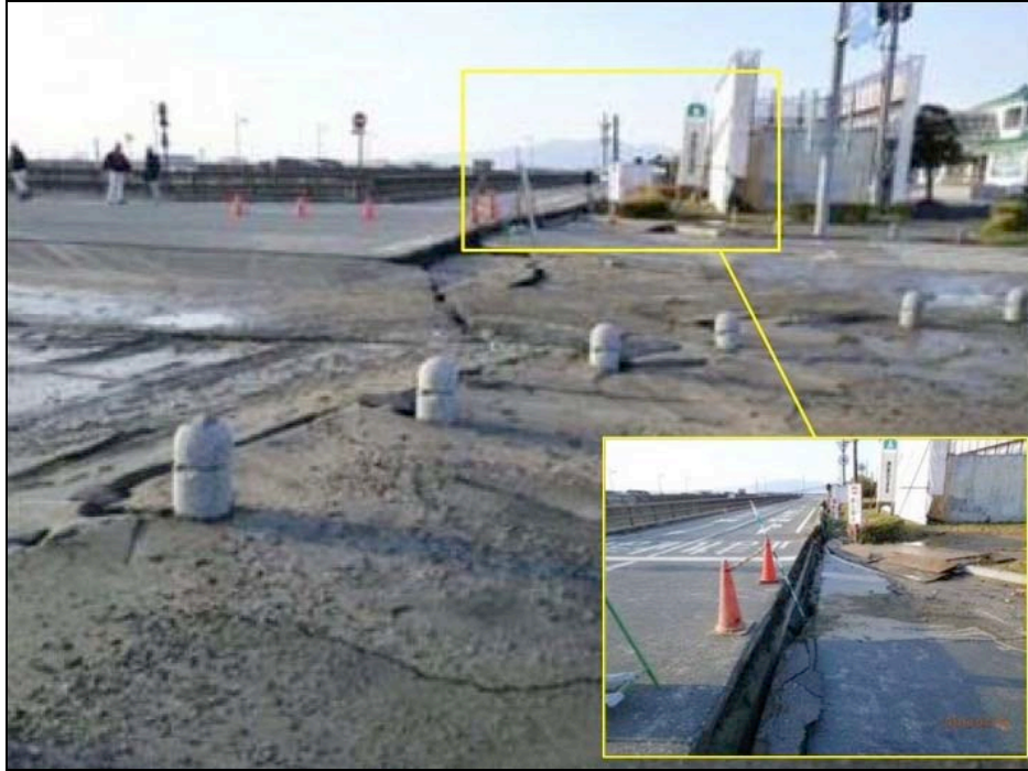
Figure 6-4. Road surface cracked and ground settlement – Kumamoto Port (Source: Kumamoto Prefecture, Civil Engineering Department)
