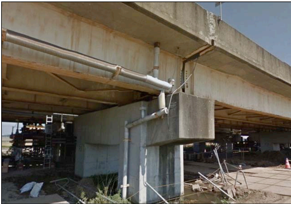
Figure 9-19. Pounding damage to both concrete side wall and junction plate of the steel girder (Tang)
