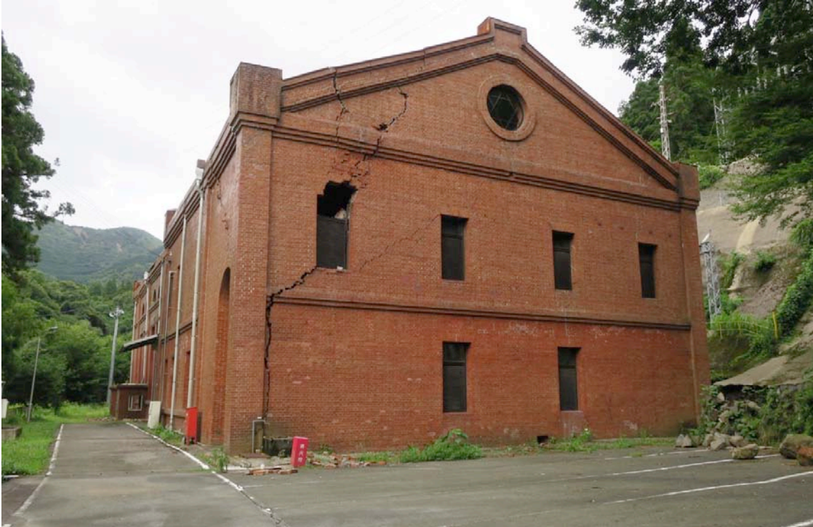
Figure 3-49. Damage at the JNC Hydroelectric Plant
