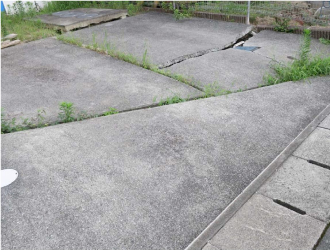
Figure 2-36. Driveway damaged by liquefaction
