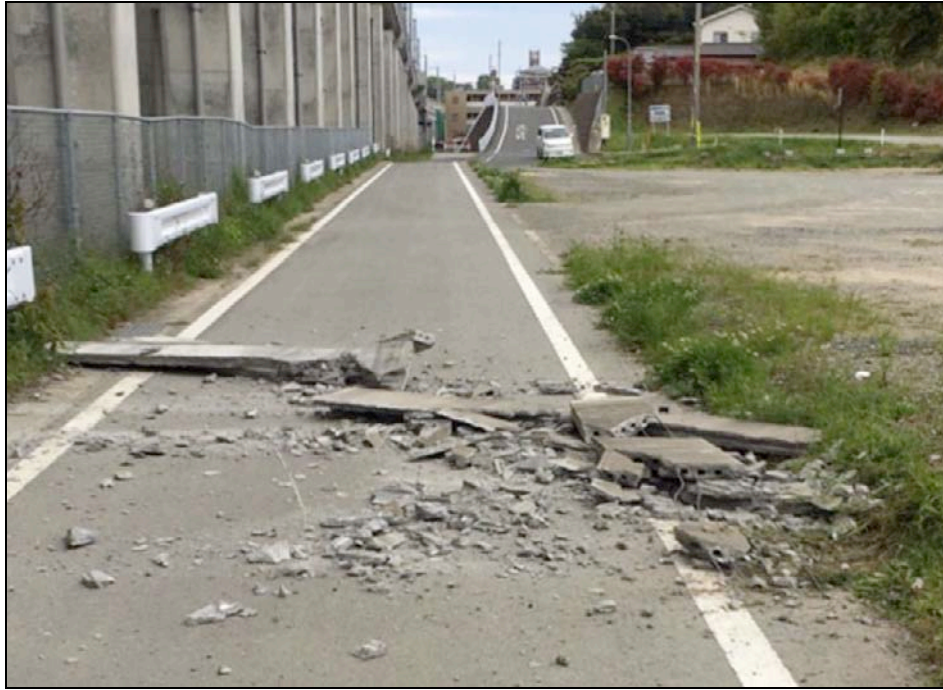
Figure 9-77 The sound barrier of the raised track fell to the ground
