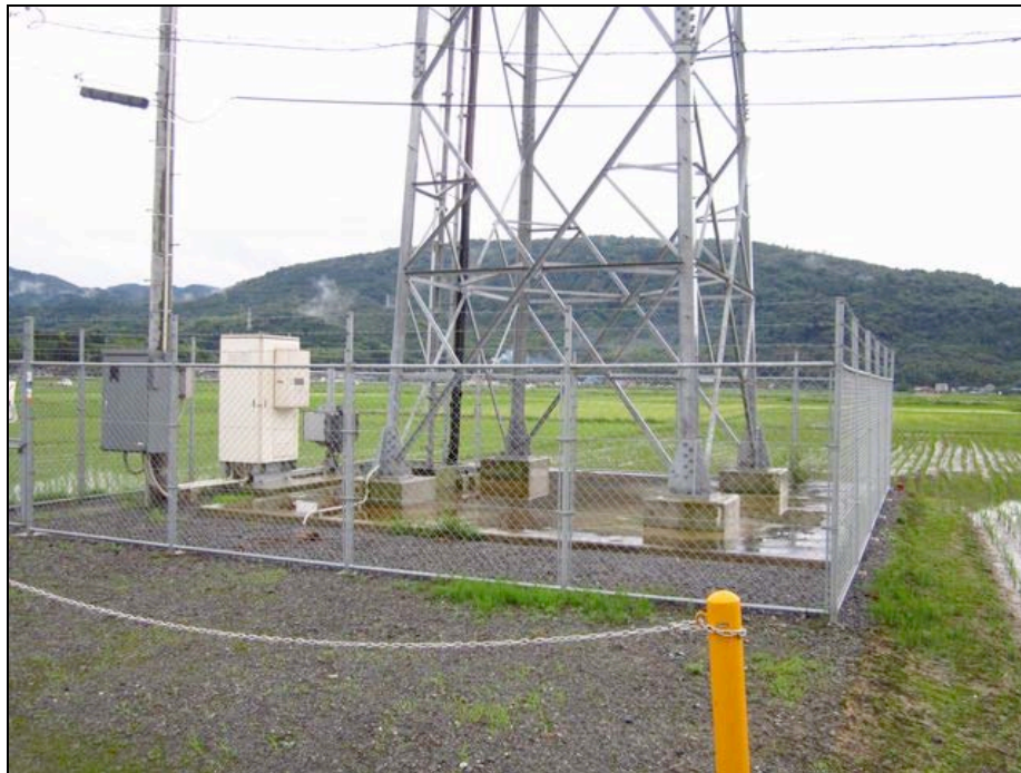
Figure 4-24. Close up view of the cell site in Figure 4-23 shows that the equipment is only about 0.5 meter above the field level
