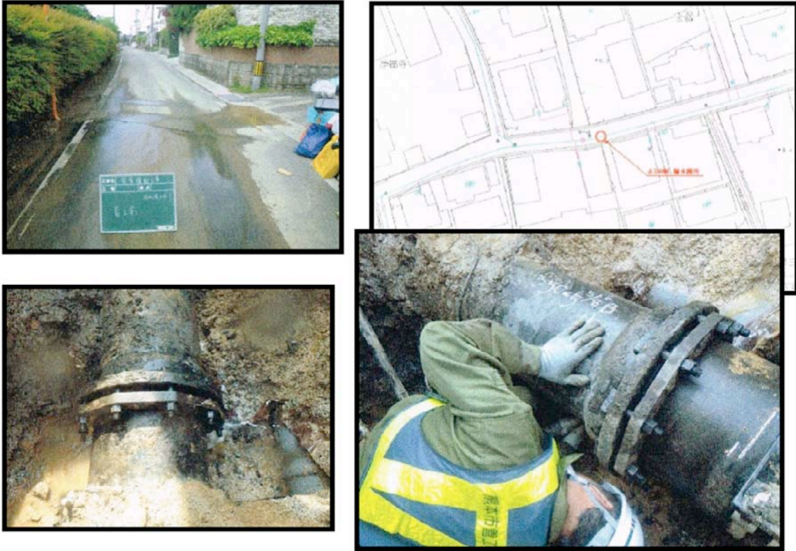
Figure 5-18. Leak of 350 mm (14-inch) cast iron pipe, near Sanchome Numayamazu
