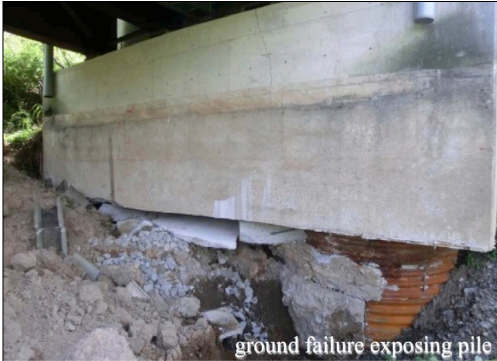
Figure 9-44. Ground failure close to the abutment support, the pile was exposed
