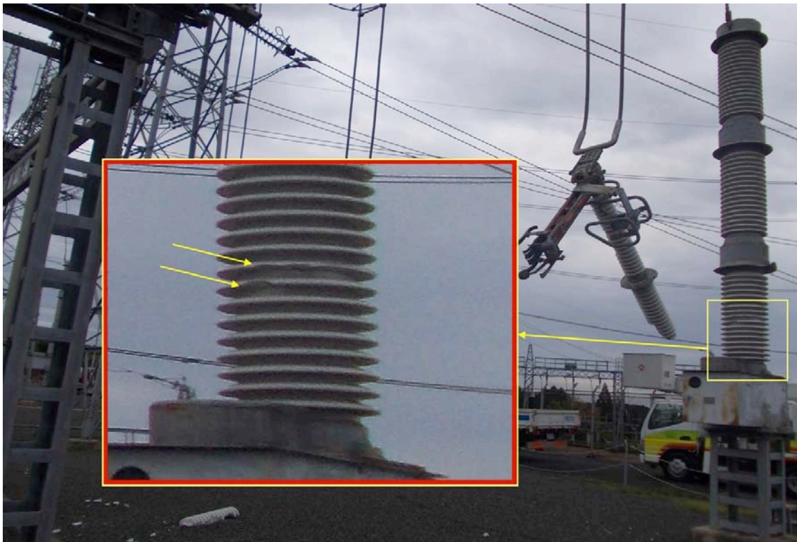
Figure 3-35. Damaged VT and DS 1 in 220 kV Yard
