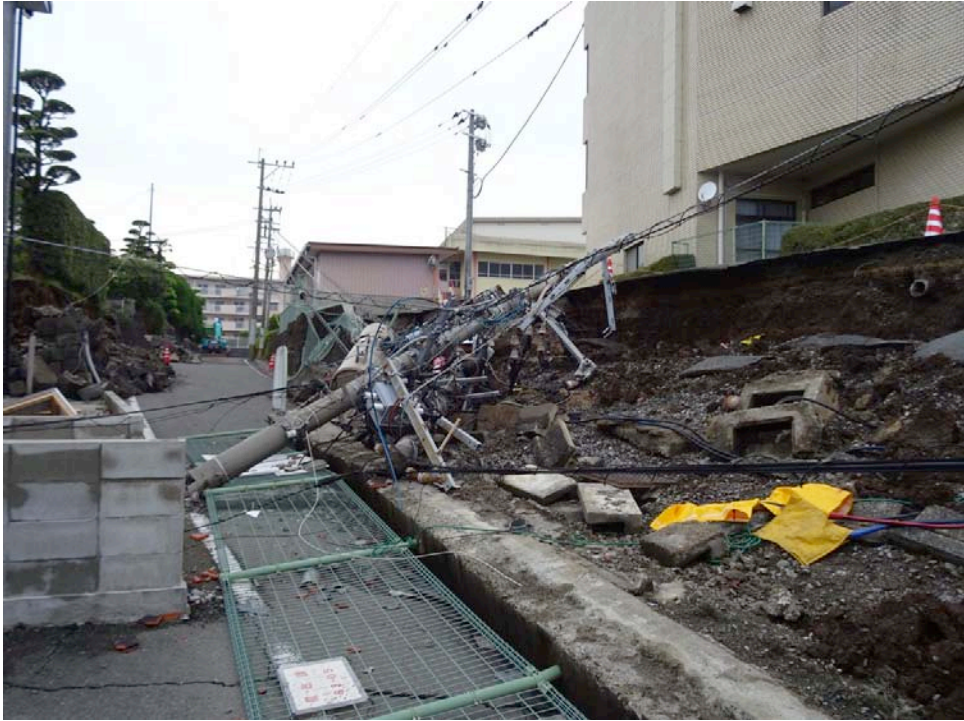
Figure 3-53. Distribution Pole Collapse
