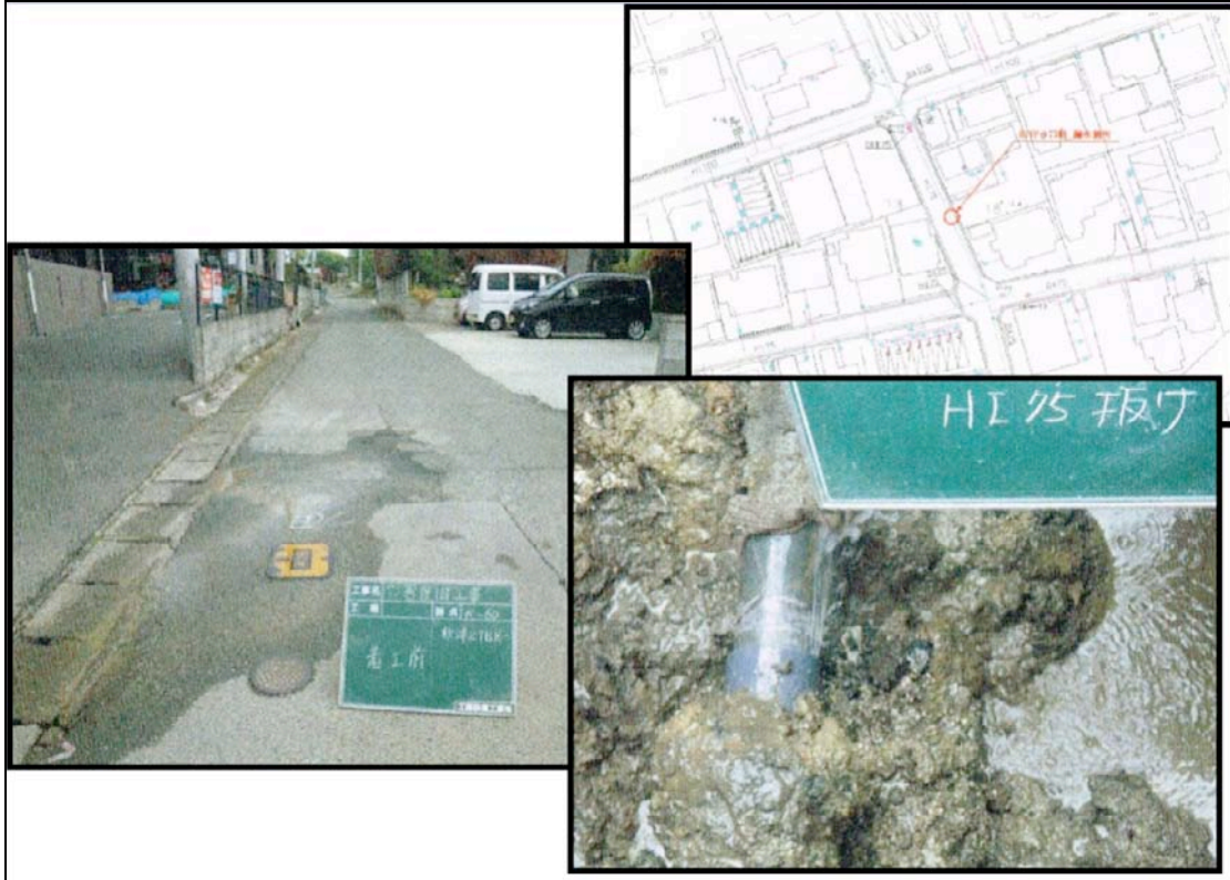
Figure 5-16. Leak of 3-inch High Impact PVC (HIVP) Pipe, near Nichome Akitsu
