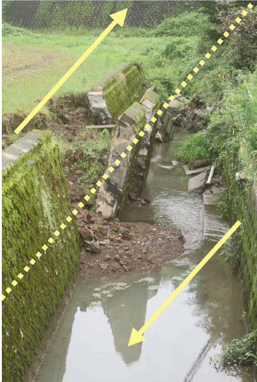
Figure 2-28. Surface faulting through concrete-lined irrigation channel
