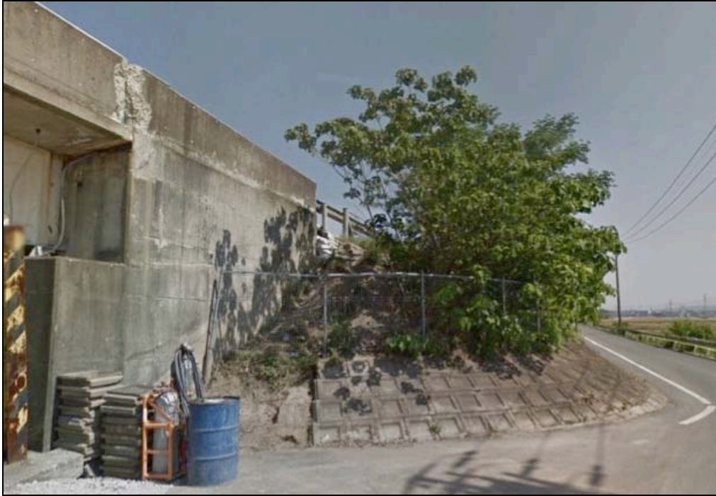
Figure 9-18. Pounding damage to side rail at the abutment (Tang)
