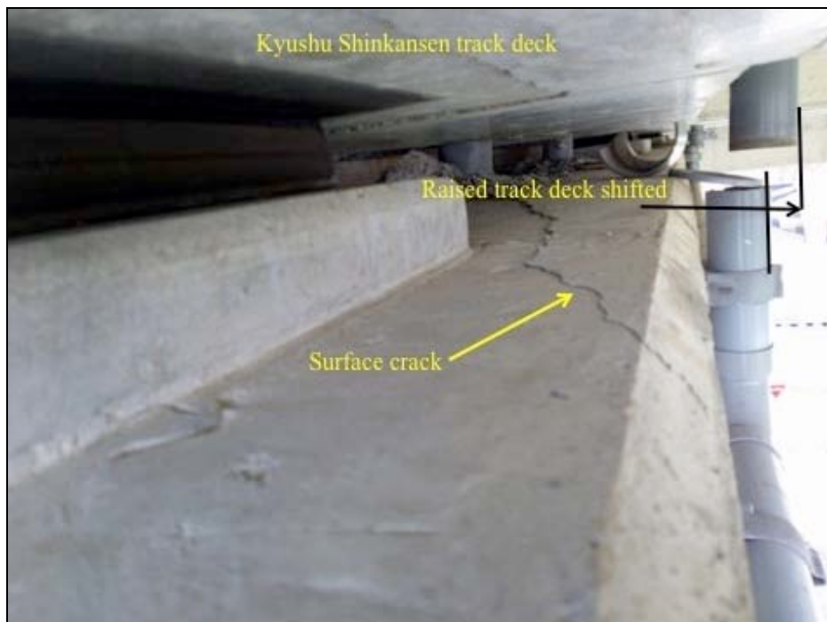
Figure 9-76. The rail platform shifted and broke the drain pipe. The concrete surface also showed cracks. Note the bearing is very close to the edge of the support
