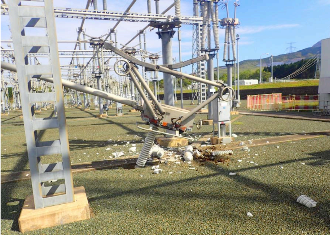
Figure 3-38. Damaged Pantograph Switch DS 5 in 220 kV Yard
