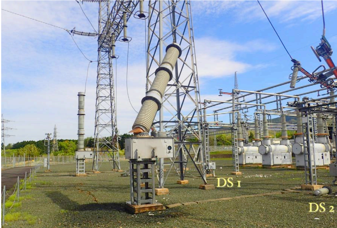
Figure 3-34. Damaged VT and DS 1 and DS2 in 220 kV Yard
