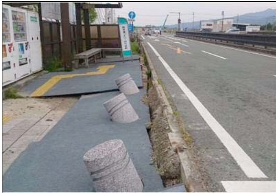
Figure 6-6. Ground settlement - Yatsushiro Port (Source: Kumamoto Prefecture, Civil Engineering Department)
