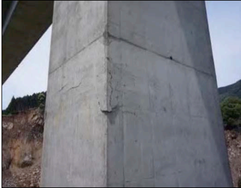
Figure 9-50. P2 pier close to the base showed concrete spalling
