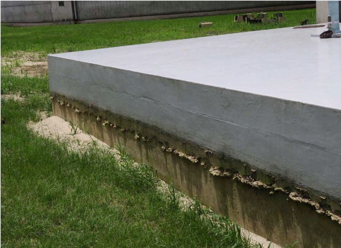
Figure 5-36. Buried Vault Soil Settlement
