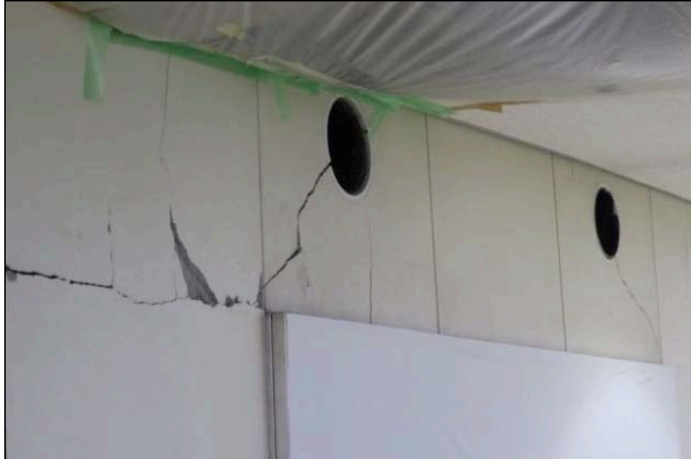
Figure 7-7. Cracks along the upper part of this dry wall
