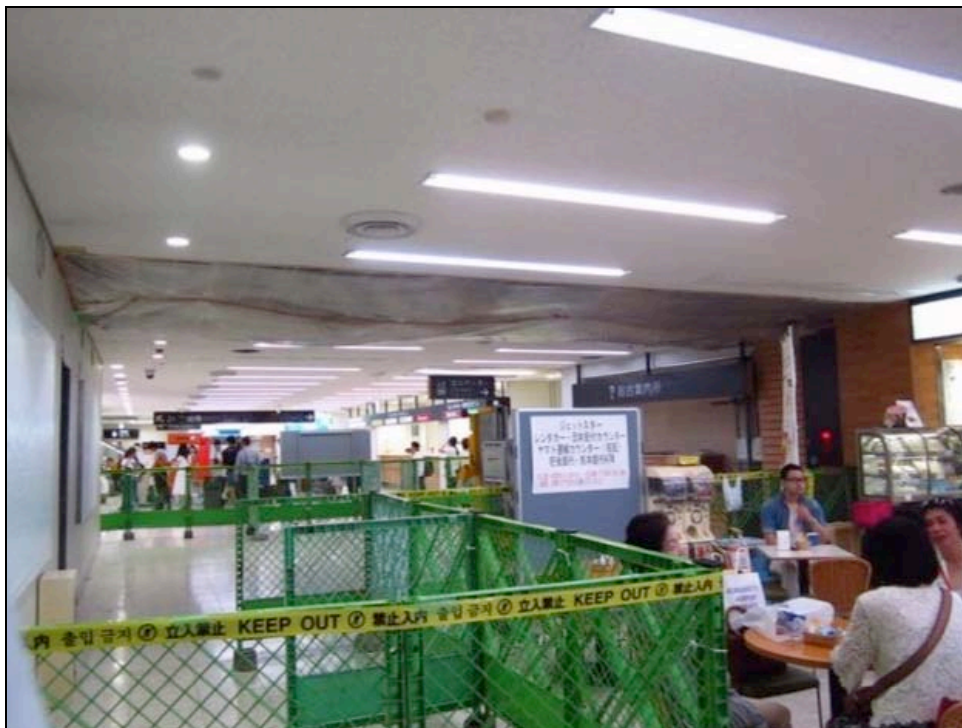
Figure 7-6. Ceiling damaged in the concession area, which was closed on July 3 2016
