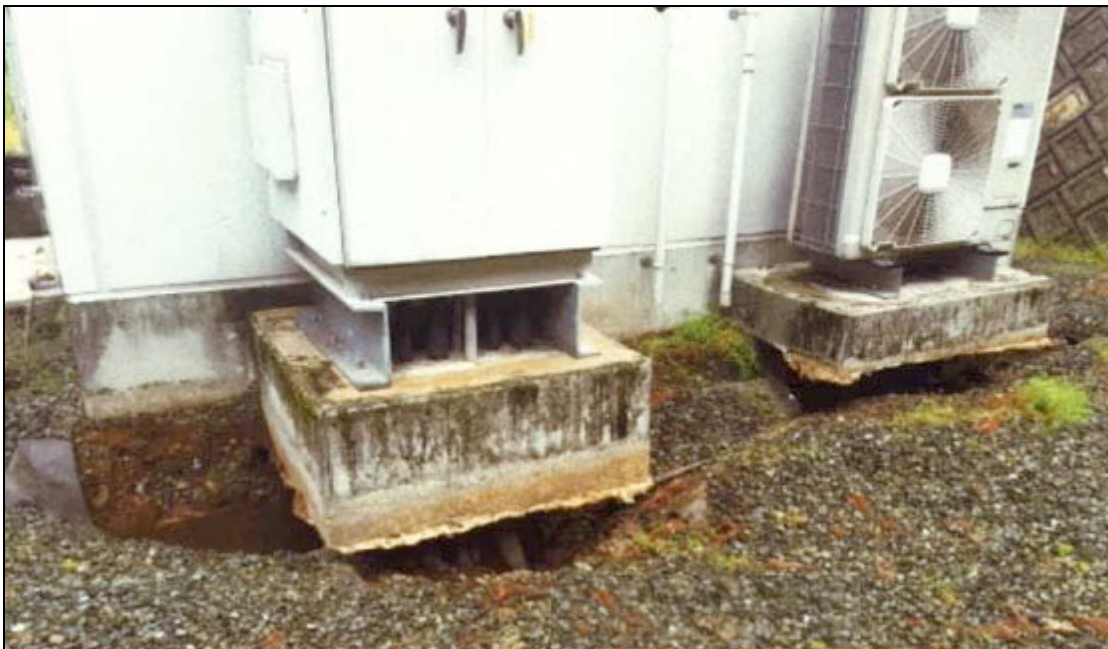
Figure 4-13. The transmission link at this cell site was damaged by the ground subsidence. (Courtesy: NTT West)
