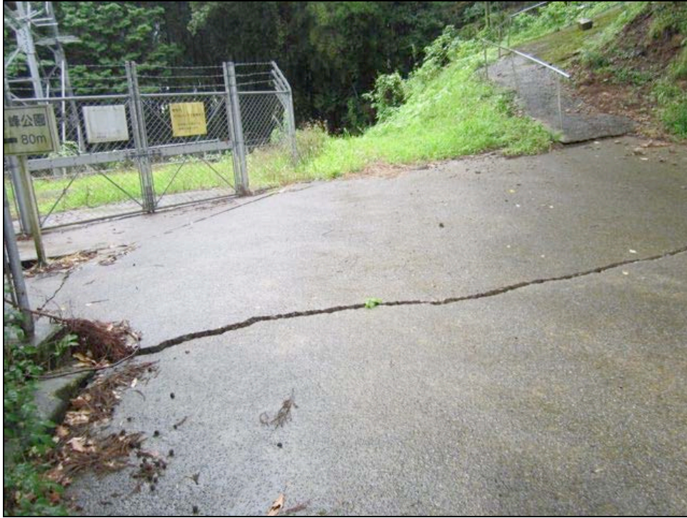
Figure 4-18. Two cracks were visible just in front of the cell site gate.
