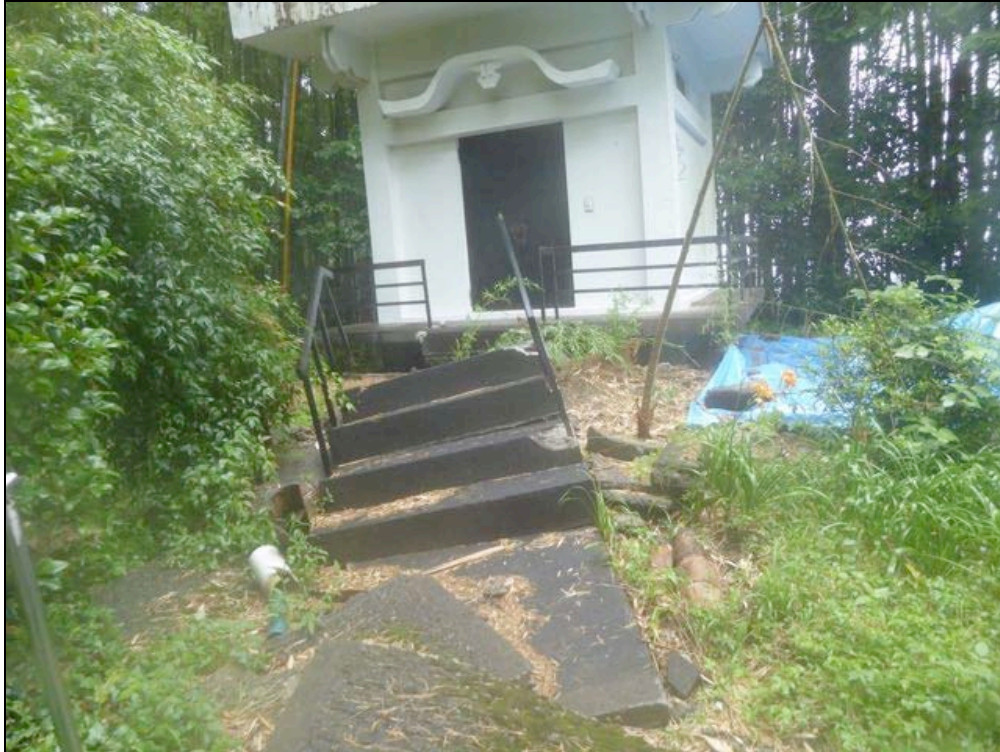
Figure 4-22. This concrete path with step to the small shrine sustained damage due to ground deformation. This shrine is about 10 meters above the cell site. The cell site aerial photo was taken from this point
