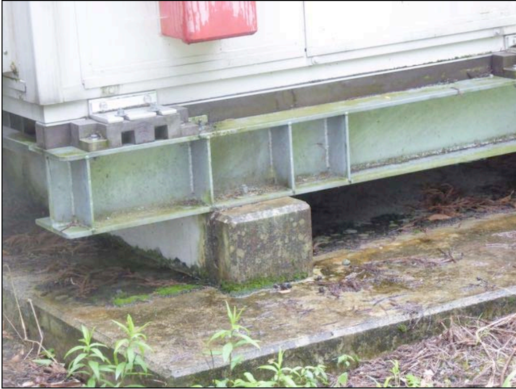
Figure 4-20. The equipment hut anchoring does not show any stress or deformation. The concrete pad was in good shape
