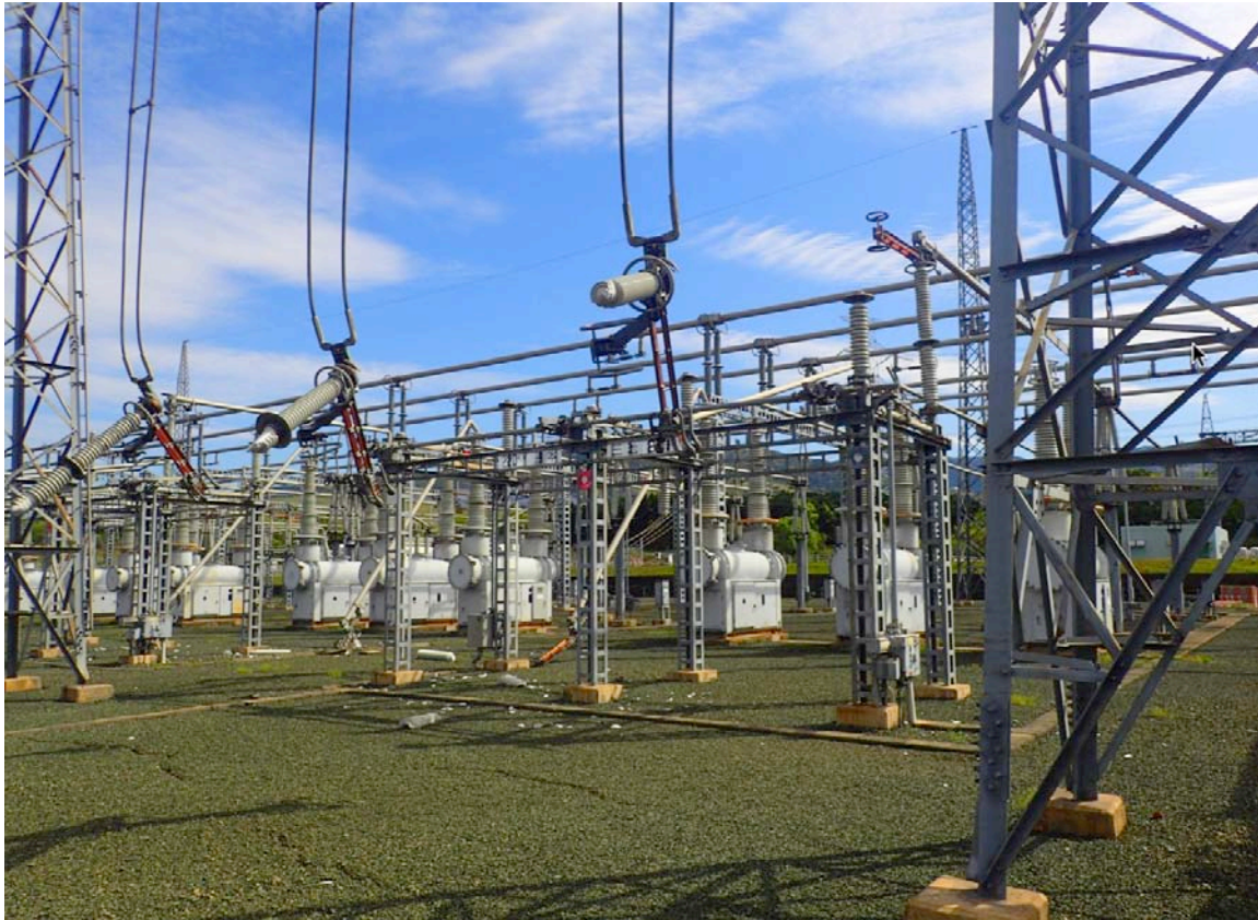
Figure 3-36. Damaged DS 4 in 220 kV Yard
