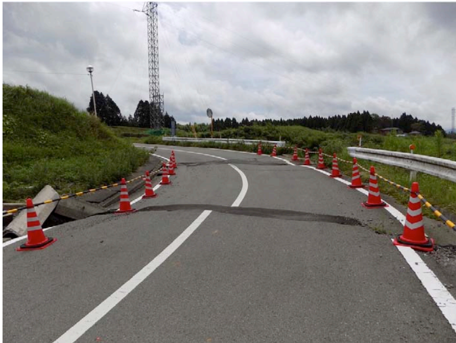
Figure 9-63. The cracks were filled with asphalt to allow traffic flow. This section of road was exposed to surface faulting. Note the destroyed surface water drain on the left side of the road has not yet been repaired. (Tang)
