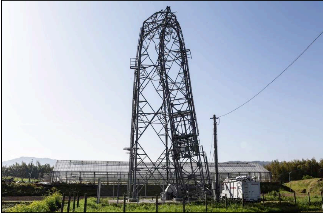
Figure 4-11. Collapsed cell tower (Courtesy: Guardian News & Media Ltd)
