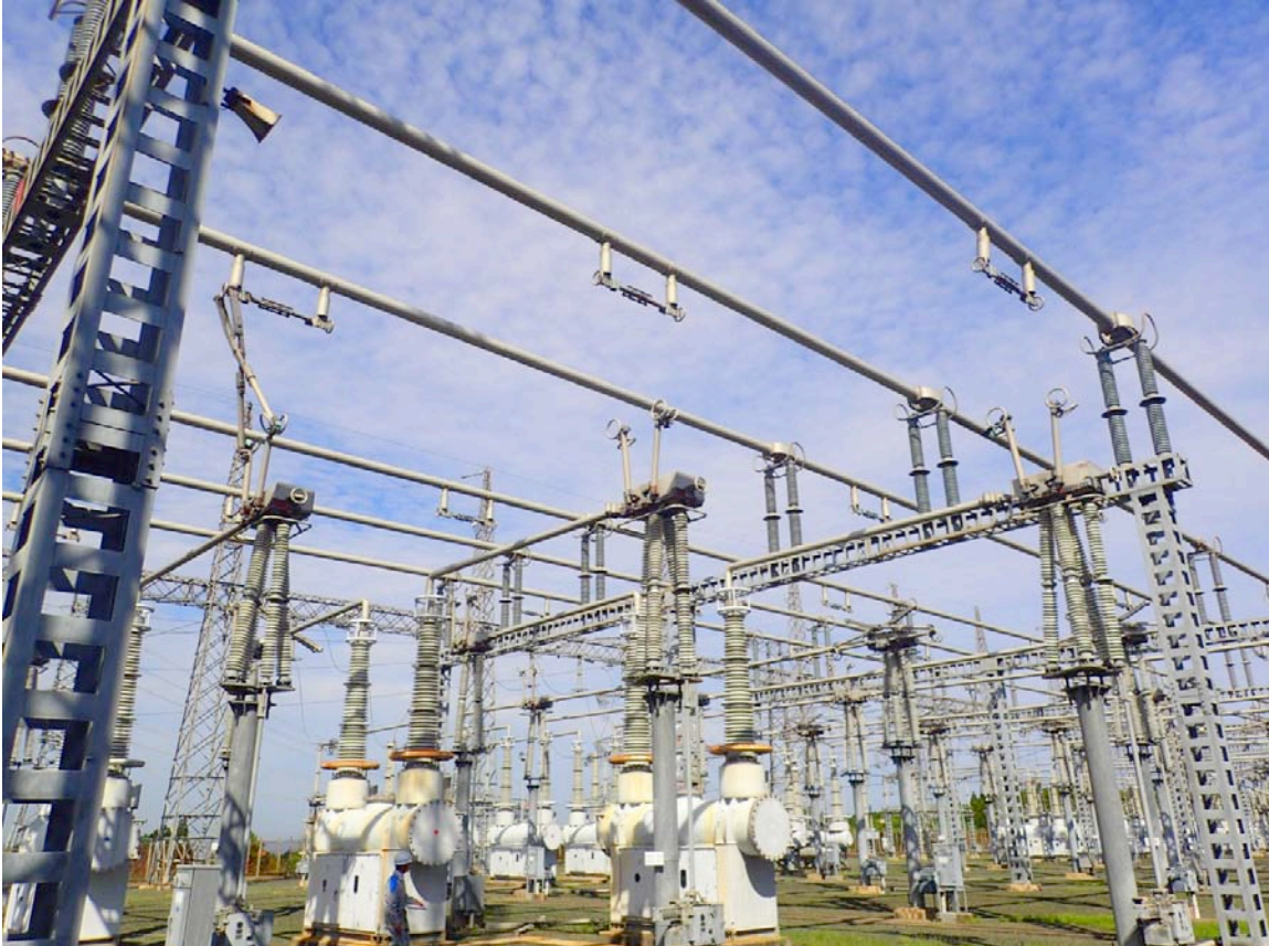
Figure 3-37. Damaged Pantograph Switch DS 5 in 220 kV Yard
