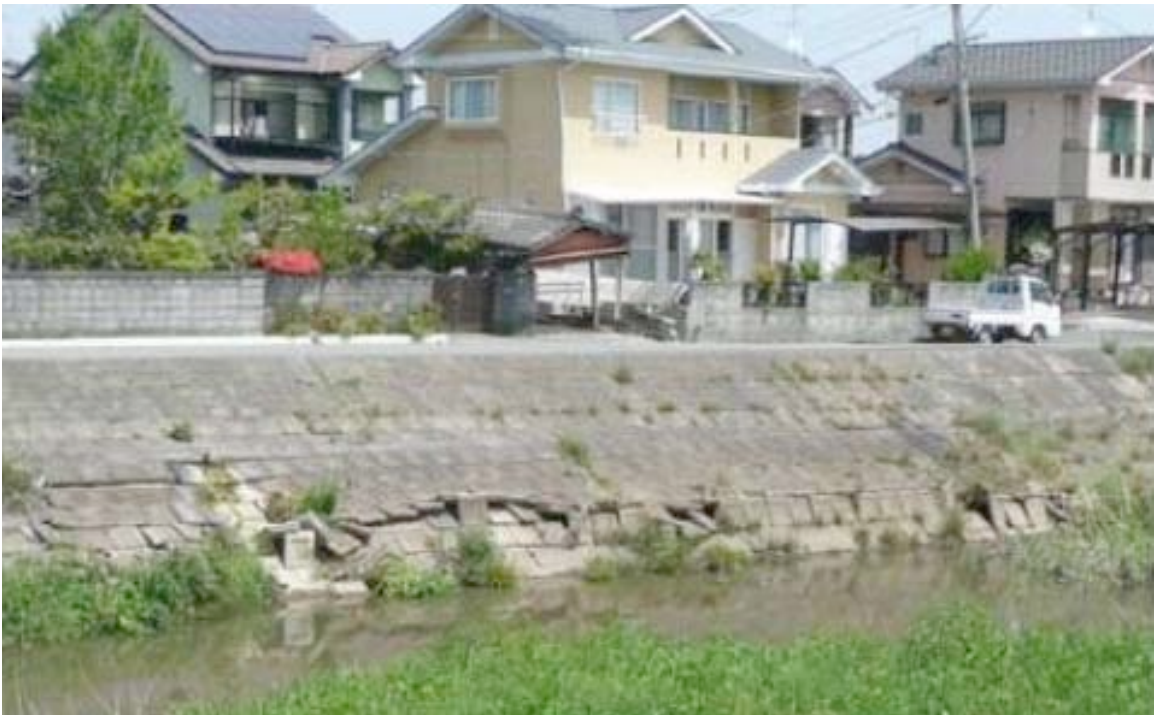
Figure 10-4. Levee Damage. Akitsugawa River (Masuki-cho). Seawall collapse
