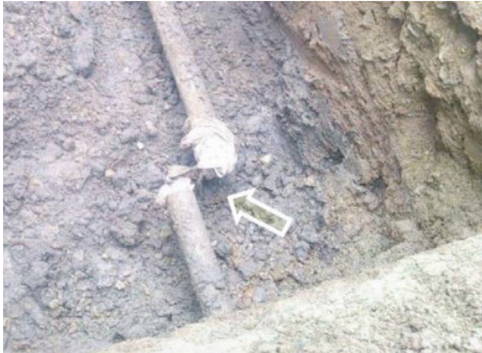
Figure 8-12. Damaged at Screwed Joint for Low Pressure Distribution Pipe (typical of 46 locations)
