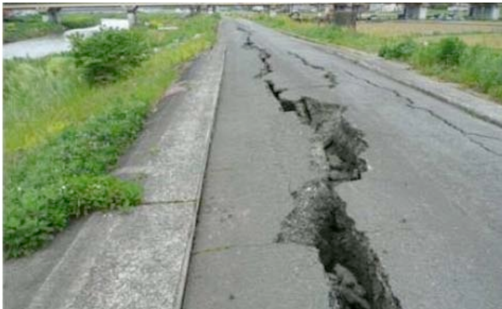
Figure 10-2. Levee Damage. Kiyamagawa River (Masuki-machi)
