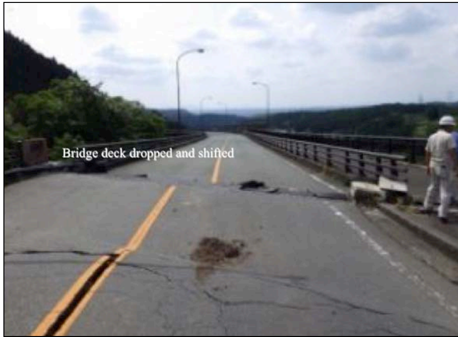
Figure 9-37. The abutment "appears" raised as the bridge deck shifted sideways off its rubber bearings and fell on the abutments
