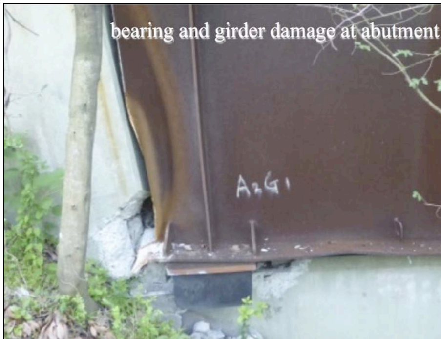
Figure 9-45. Damage to the abutment concrete and the bearing pad as well as the steel girder
