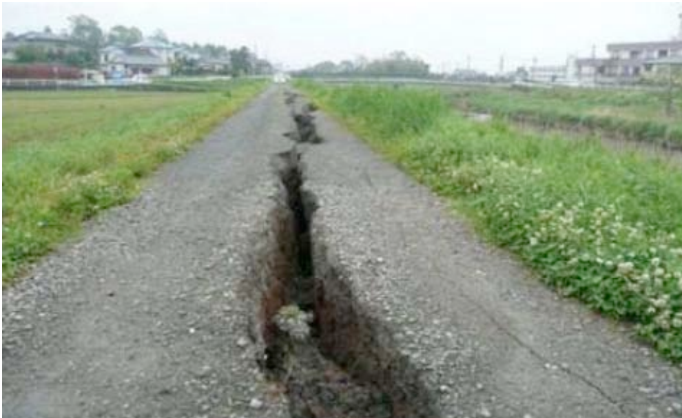
Figure 10-1. Levee Damage. Yagata River (Masuki-machi)
