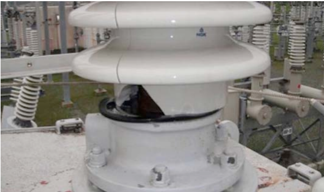
Figure 3-45. Damaged T Bushing for 66 kV Shunt Reactor in Figure 3-43
