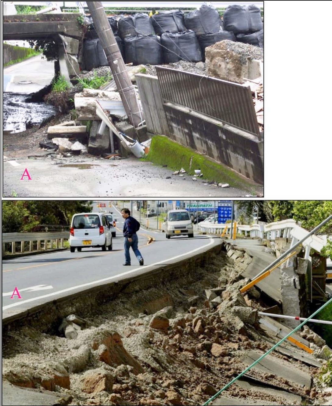
Figure 9-57. The embankment failure and temporary fix of (A)
