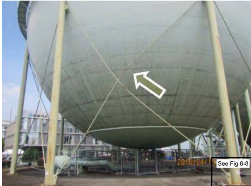
Figure 8-7. Gas Holder with Yielding Cross Braces
