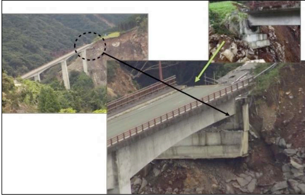
Figure 9-48. West end of the bridge, damage to the abutment and bridge deck
