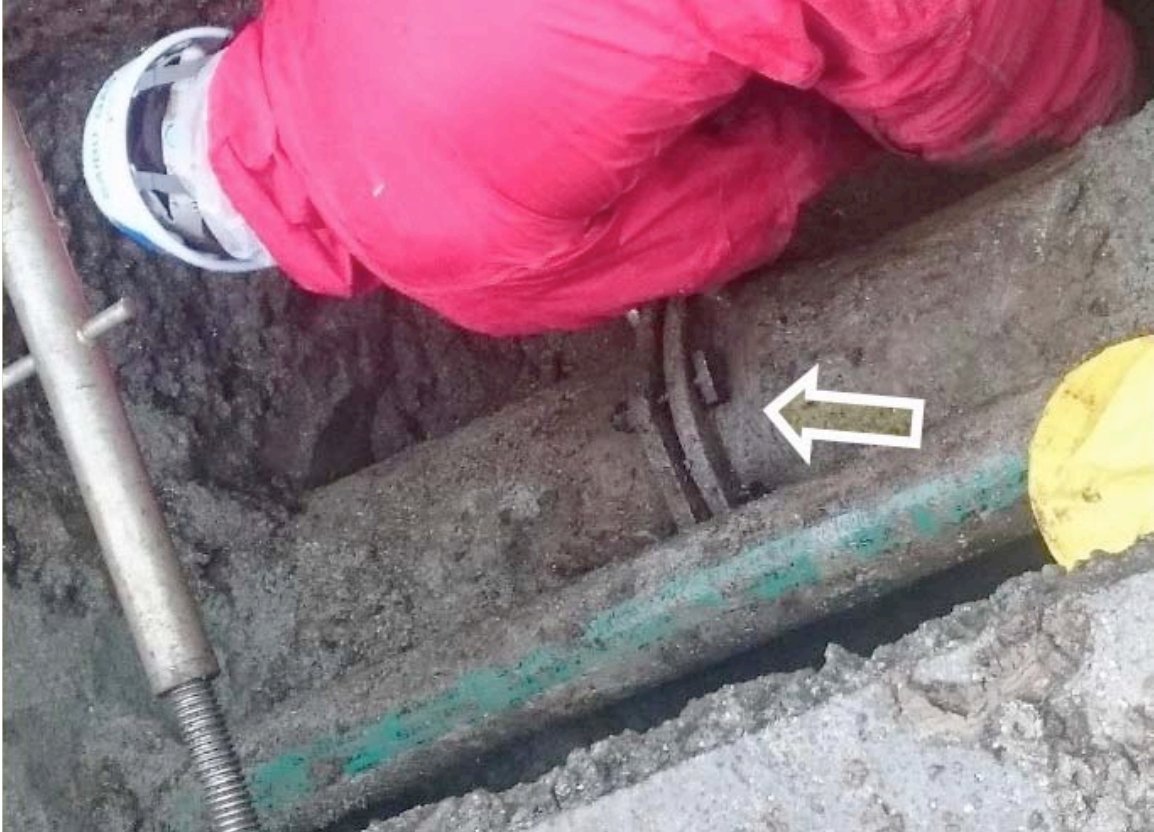
Figure 8-10. Repair to Median Pressure Class B Pipe. Repair was to tighten the mechanical joint (typical of 9 locations)
