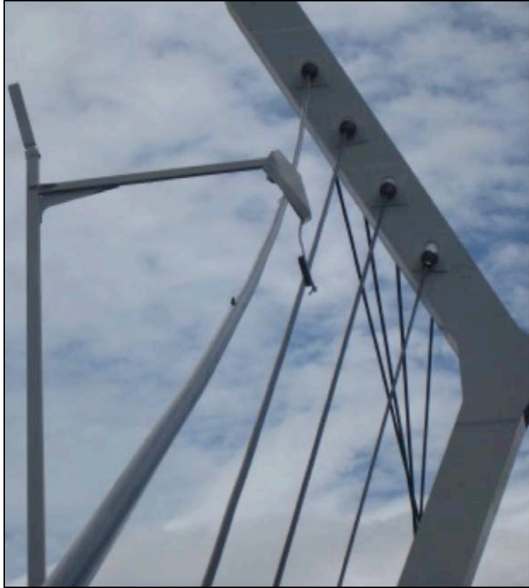
Figure 9-41. A few cables were loose
