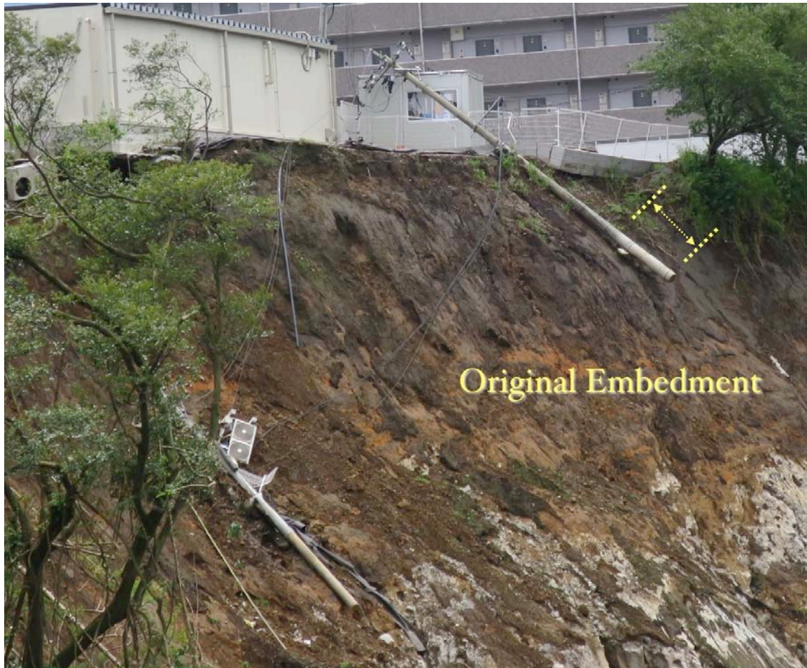
Figure 2-25. Slope Failure with Distribution Pole
