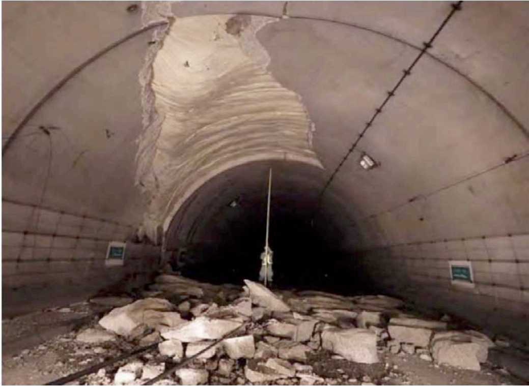
Figure 9-67. Tunnel cladding broke off, these were very large pieces of concrete
