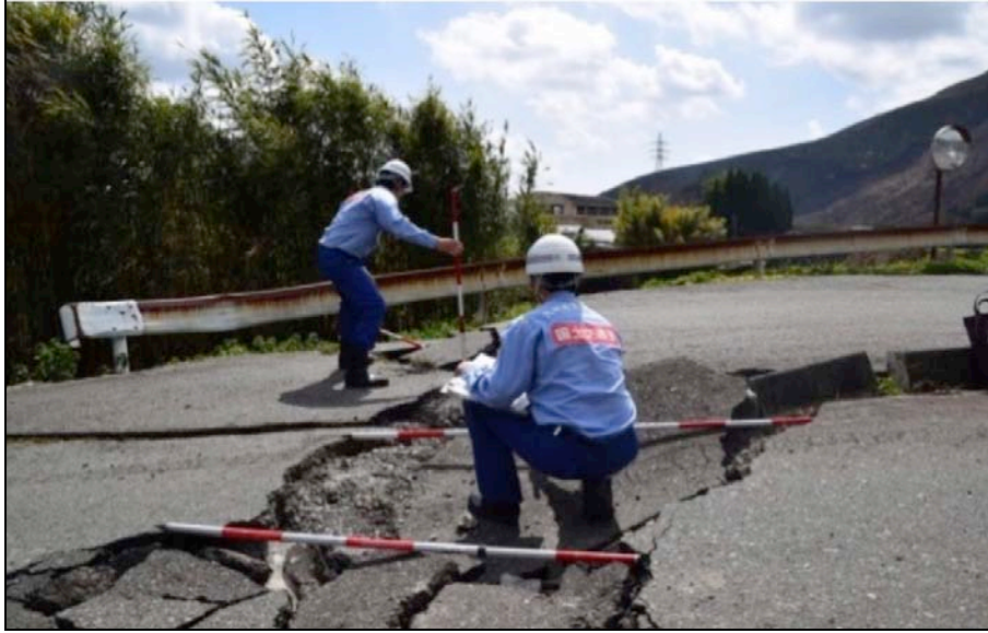
Figure 9-95 TEC-FORCE inspecting and recording damage to Prefecture Route 149 (N32.8924°, E130.9918°)
