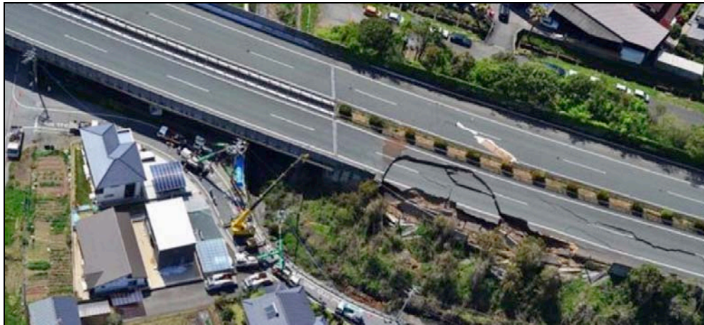
Figure 9-11. Close up view of the collapsed embankment of Kyushu Expressway
