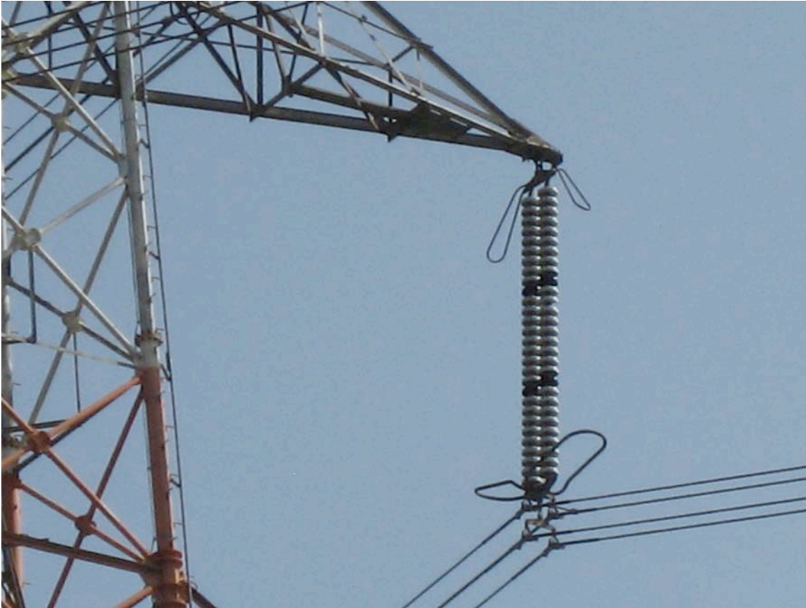
Figure 3-27. Typical 500 kV Tower Jumper Configuration, Suspension Tower
