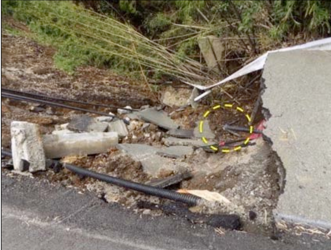
Figure 4-1. Buried cable with flexible conduit severed (Minami Aso)
