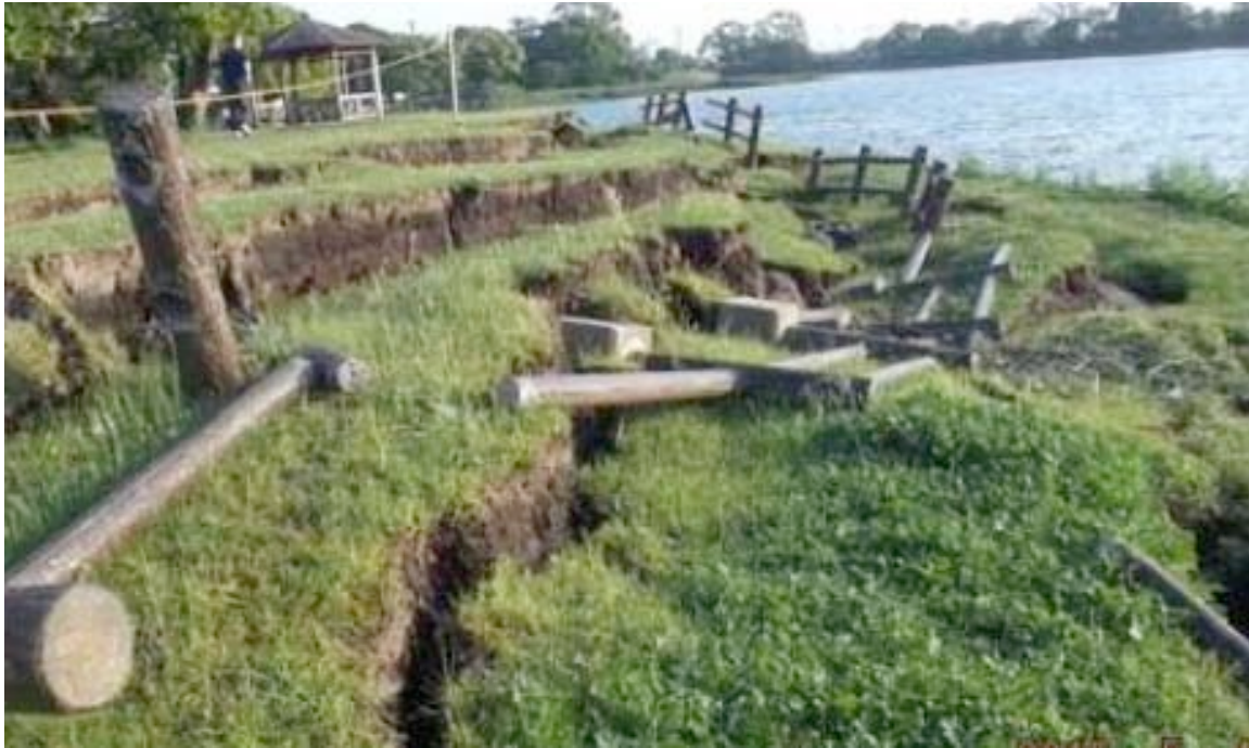
Figure 10-5. Shoreline Lateral Spread. Suizenji Ezu Lake Park, Kumamoto City
