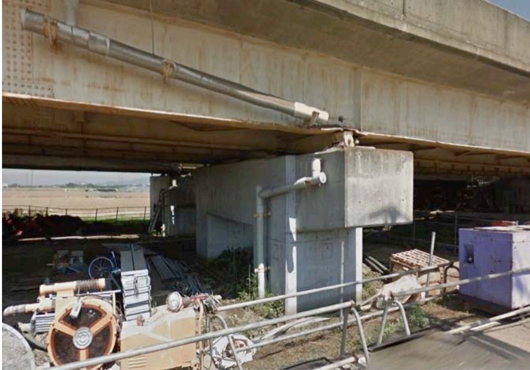
Figure 9-20. Drainpipe broken and the bearing rocker was pushed and damage the steel girder flange
