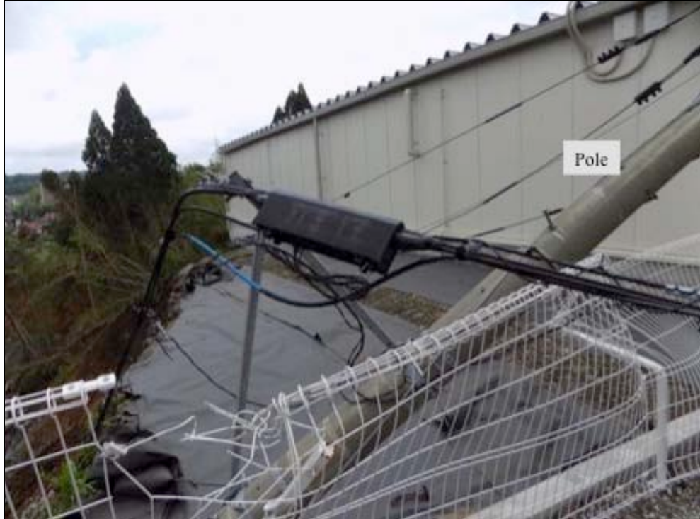
Figure 4-3. The telecom pole fell and resting on the side of the building
