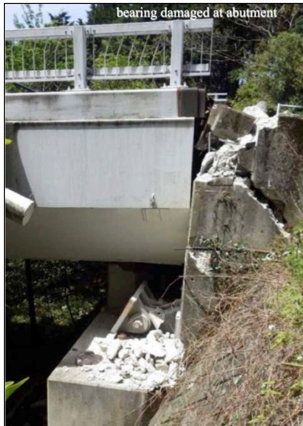
Figure 9-40. Due to pounding the bearing rocker broke off and the abutment concrete was shattered
