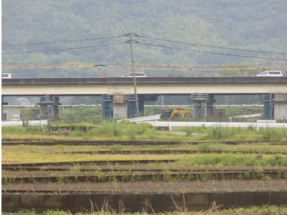
Figure 9-16. This shows another section of the bridge deck with shoring support (Tang)
