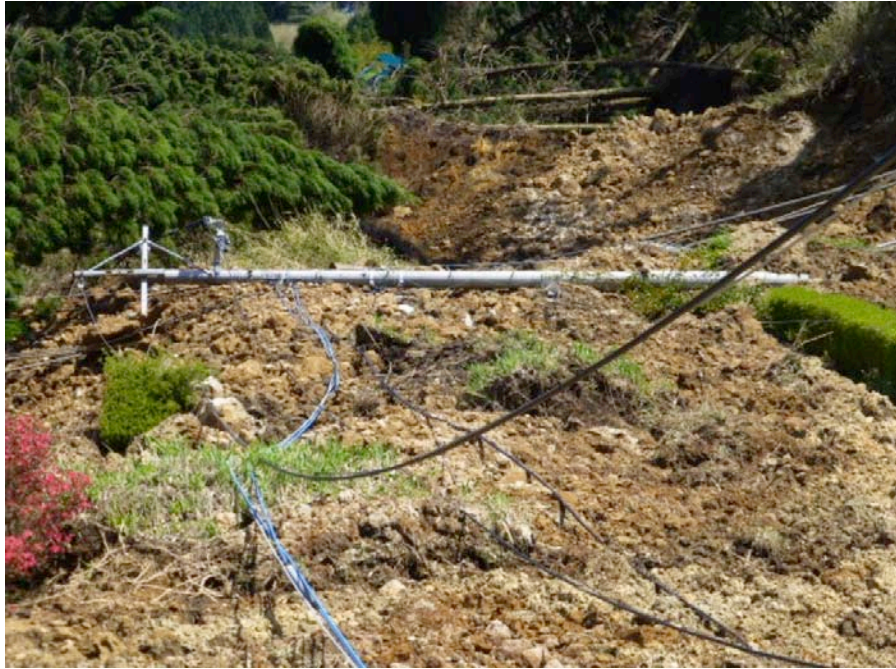
Figure 3-55. Distribution Pole Collapse
