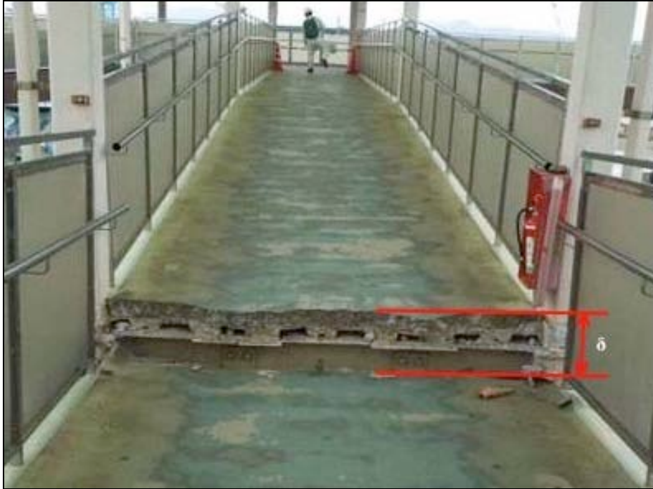
Figure 6-3. Bridge misaligned – Kumamoto Port (Source: Kumamoto Prefecture, Civil Engineering Department)
