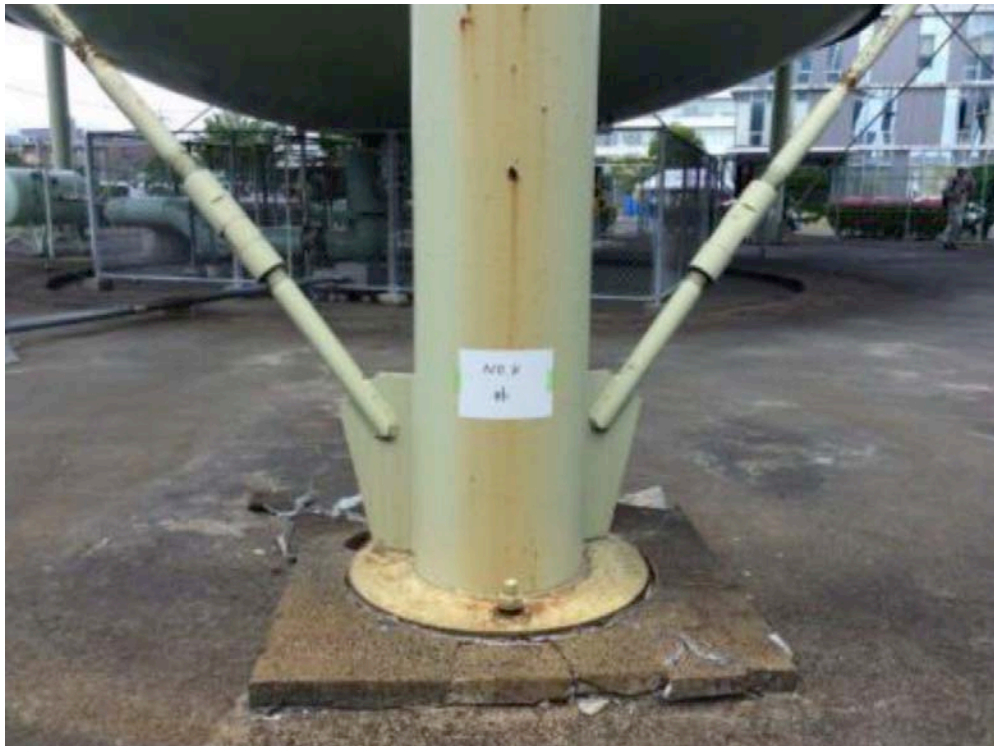
Figure 8-8. Gas Holder with Yielding Cross Braces
