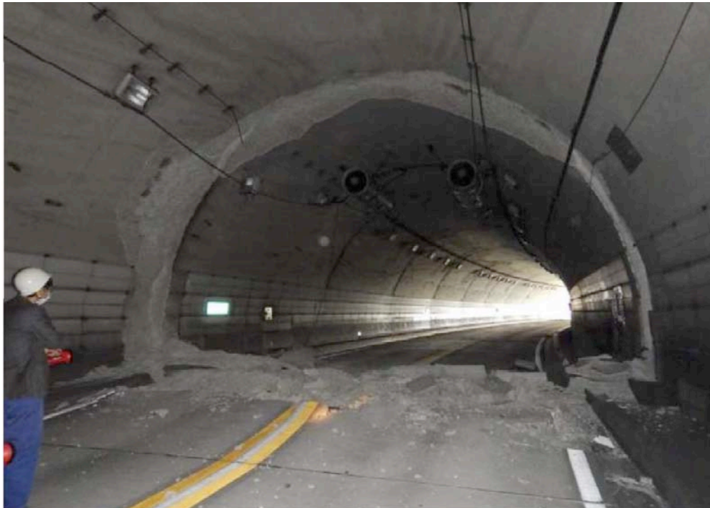
Figure 9-69. Some small piece of cladding fell and the road surface buckled
