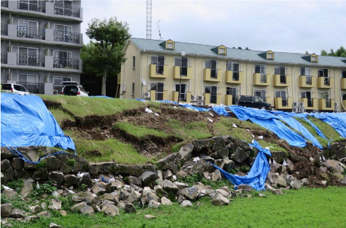
Figure 2-24. Embankment Slope Failure
