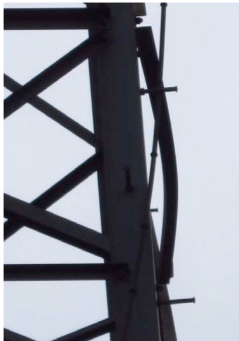
Figure 3-18. Old Tower 2 Buckle in Secondary Member
