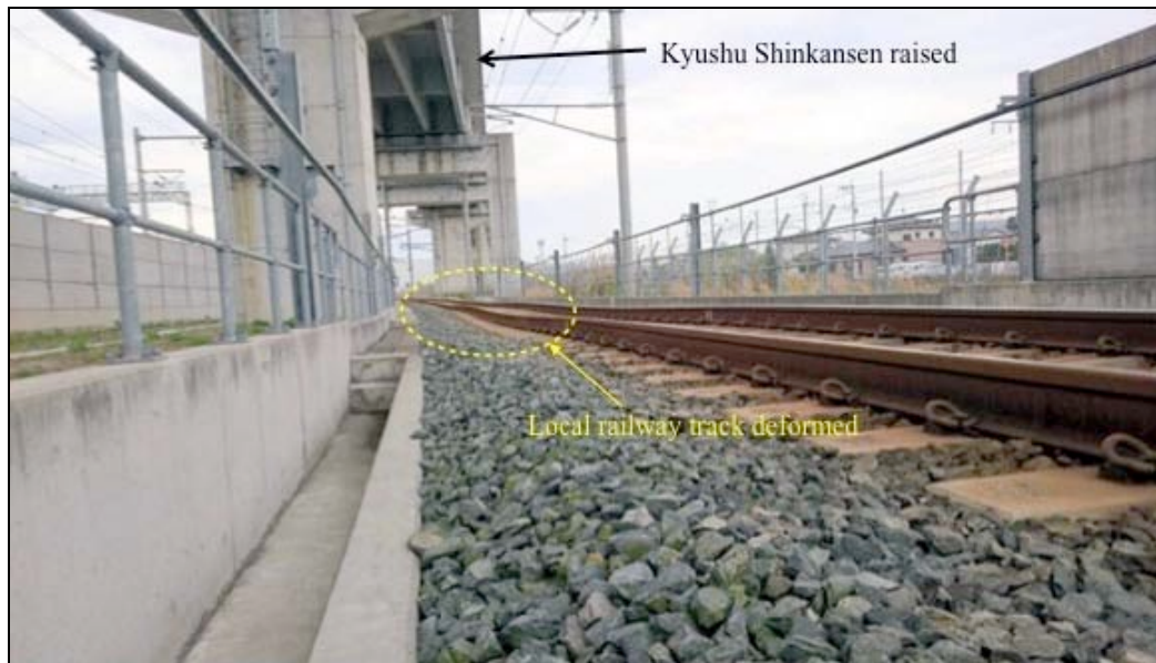
Figure 9-80. This section of JR tracks were deformed
