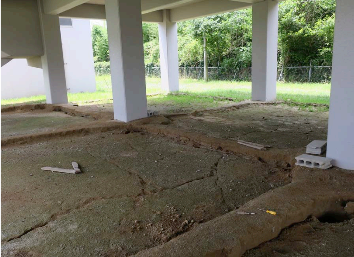
Figure 5-35. Pump Station Building Soil Settlement
