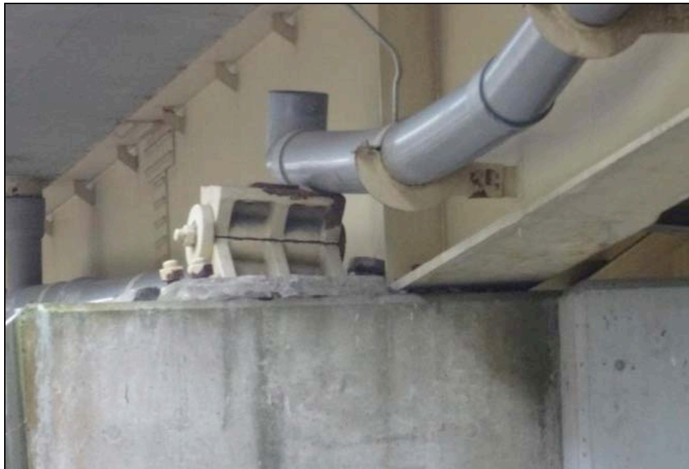
Figure 9-17. Girder slipped off the bearing pad
