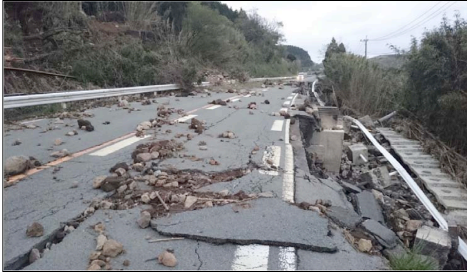
Figure 9-66. Embankment failure due to lateral spreading damage this part of Route 57
