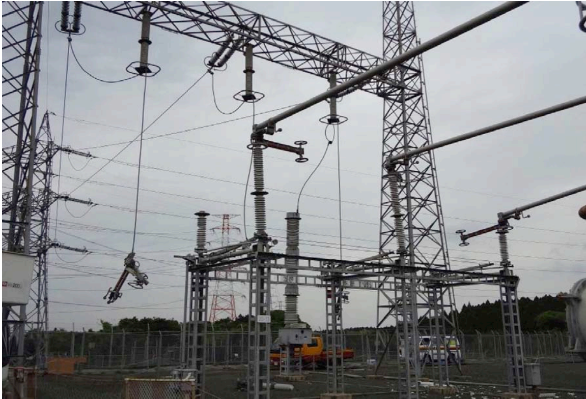
Figure 3-39. Damaged Switch DS 1 in 220 kV Yard
