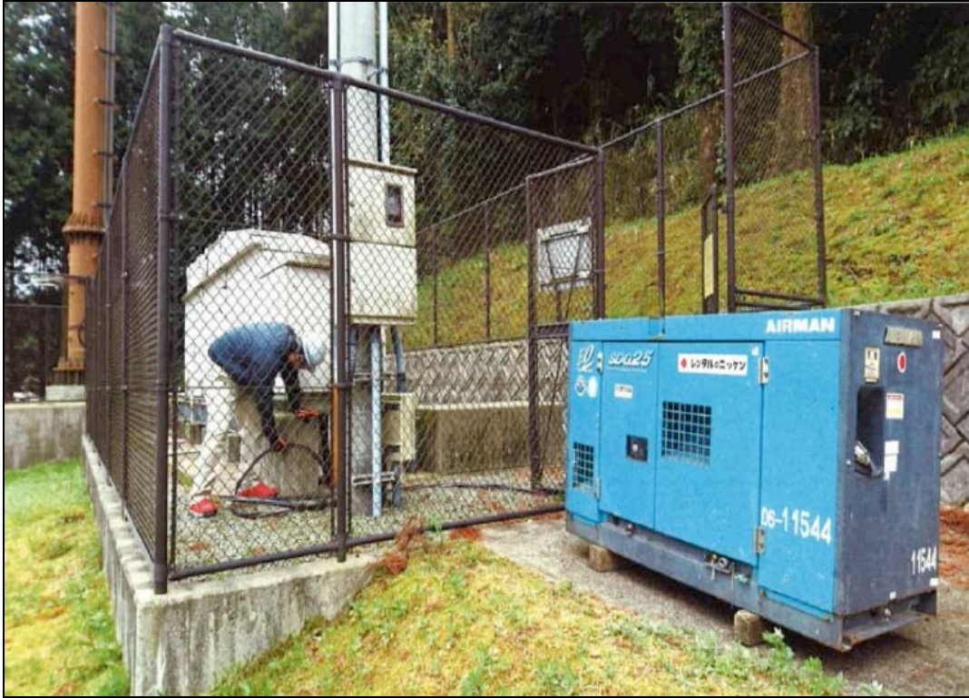
Figure 4-12. This DoCoMo Mid-zone Base Station had a power generator brought in to provide power to operate the base station. (Courtesy: NTT West)
