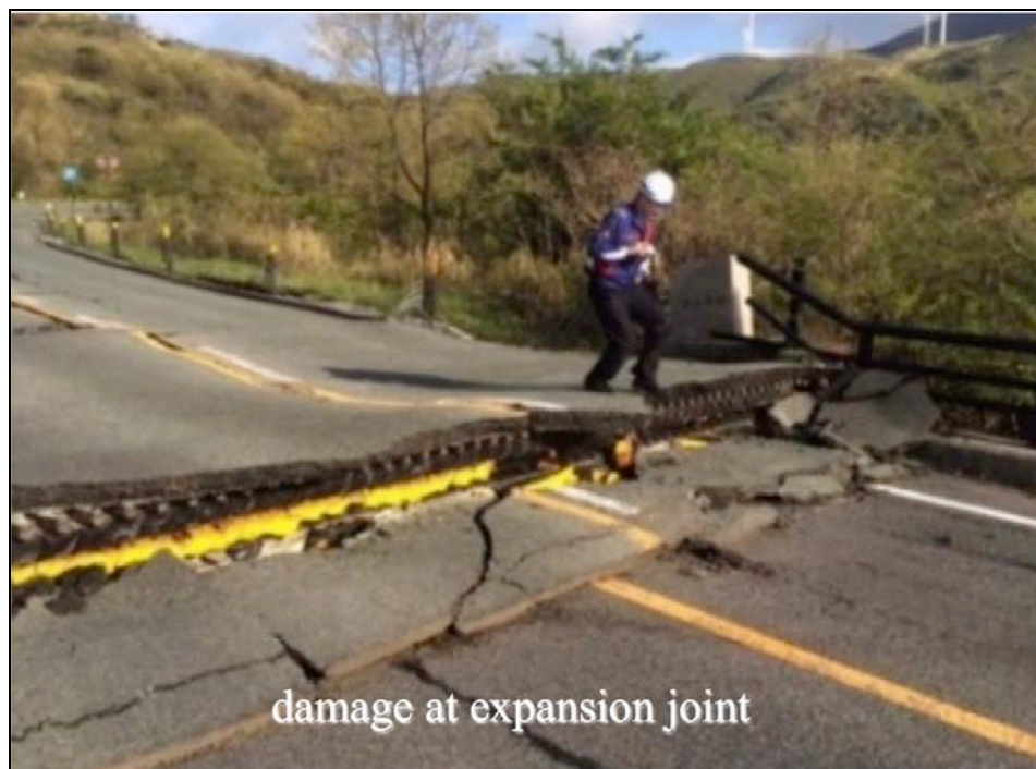
Figure 9-43. Close up view of the abutment damage at the expansion joint
