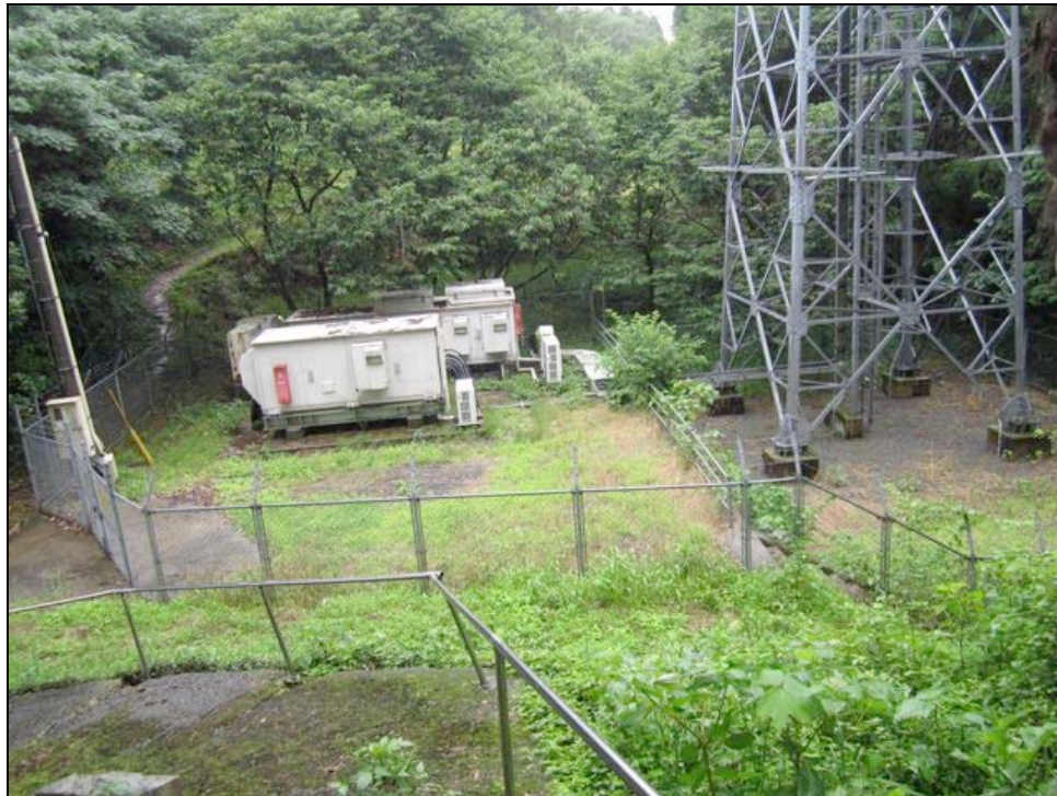
Figure 4-19. This aerial view of the cell site shows no visible damage on the outside of the huts and the tower footings
