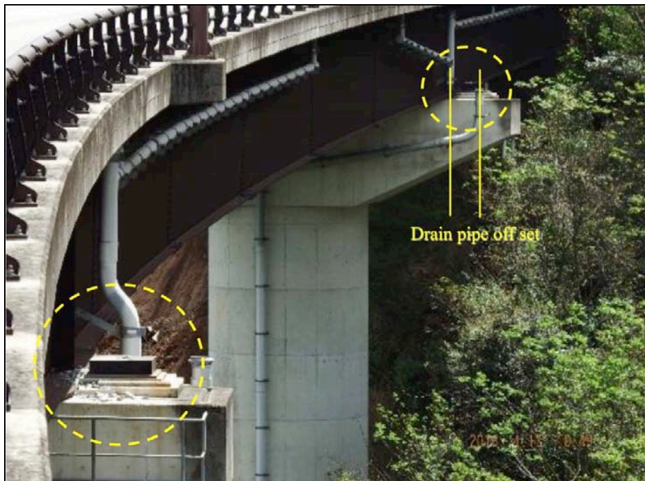
Figure 9-34. Relative movement between the deck and the support column demonstrated strong ground motion
