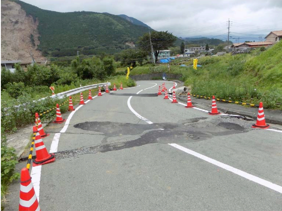
Figure 9-64. This part of road was temporarily paved to allow traffic flow (Tang)
