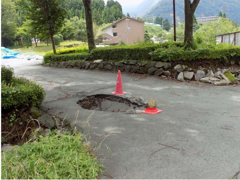
Figure 9-62. A sinkhole appeared here and it was not filled in when we were there in July (Tang)
