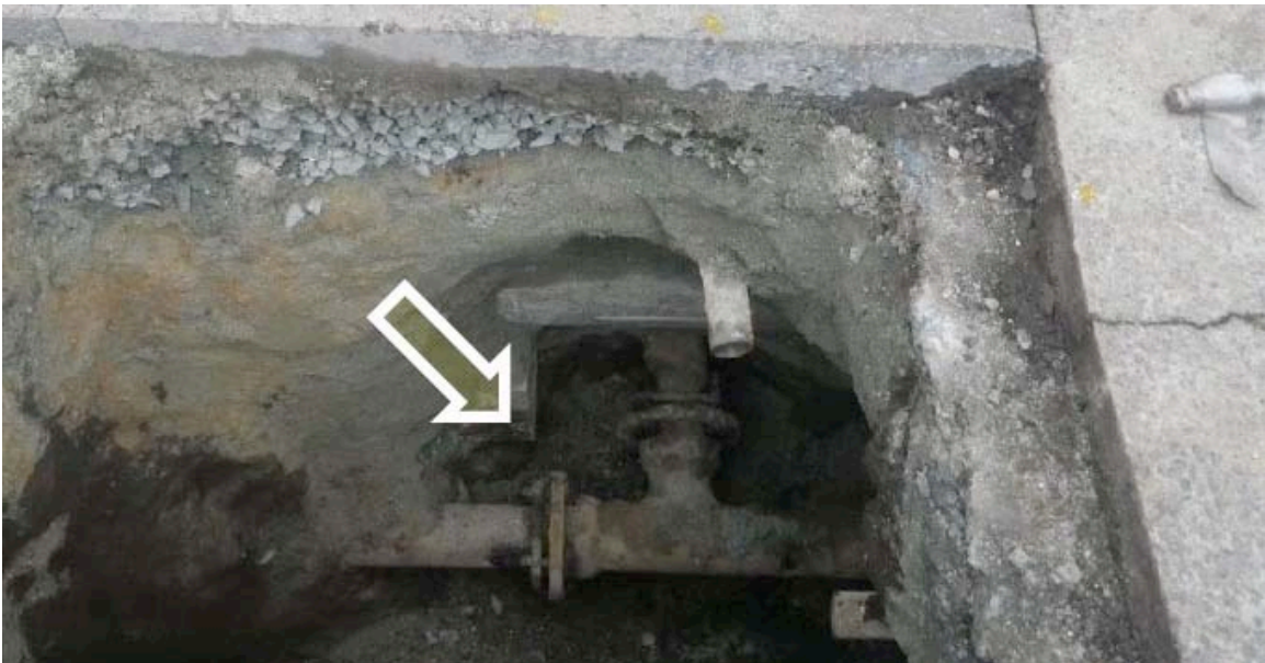
Figure 8-11. Repair to Low Pressure Distribution Pipe. Repair was to tighten the mechanical joint (typical of 23 locations)
