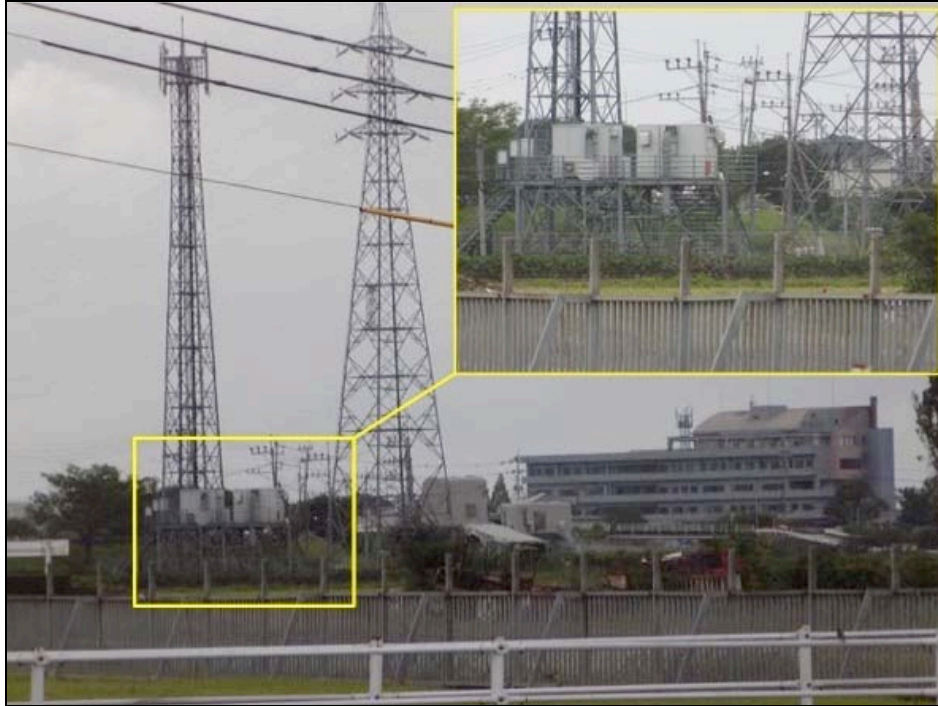
Figure 4-25. This cell site on the edge of the rice field is installed on a high steel platform. The equipment is installed with flood as one of the hazards
