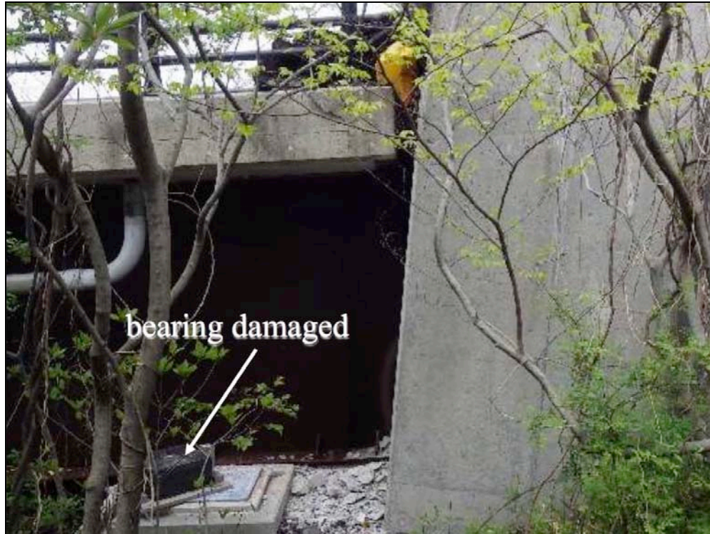
Figure 9-46. The steel girder slipped off the bearing pad
