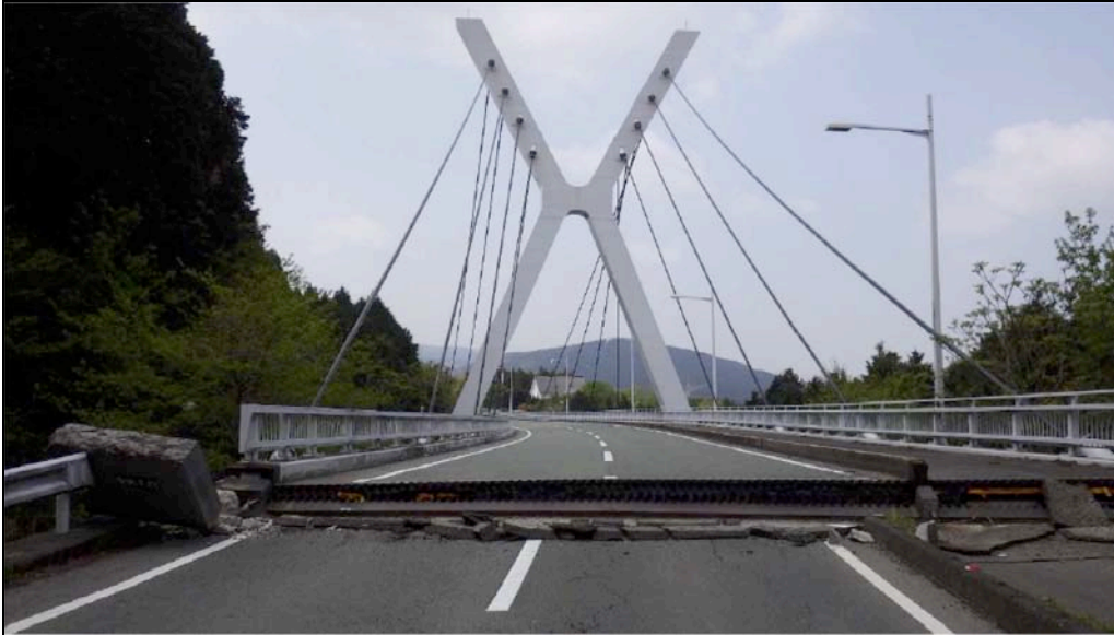
Figure 9-39. Close up view of the Northeastern abutment damage
