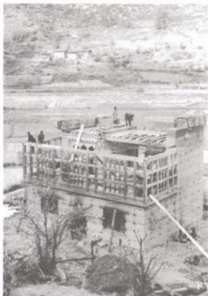
Fig. 5. Bhutan, Valley of Paro: Construction of a farm house using "pisé de terre" with a light timber framing for the upper floor.
