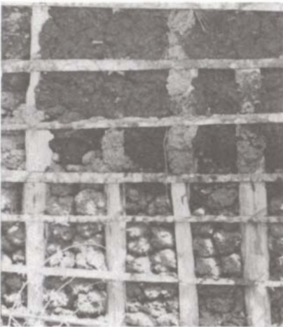
Figure 3. Balls of mud placed inside the 'pockets' of the timber frame of a wattle and daub wall; new work with wet mud is seen at the top of the picture.
