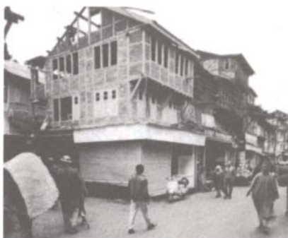
A Dhajji Dewari house being reconstructed using the traditional materials, including mud mortar. All of the exterior walls were reconstructed while the family continued to live in the house.
