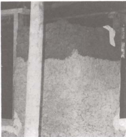
Figure 6. A section of fig. 5; the new work with wet mud looking darker than the rest of the wall, is noticeable.
