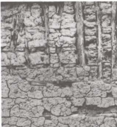
Figure 13. Decay of timber work after the loss of the mud-coat of a wattle and daub house.
