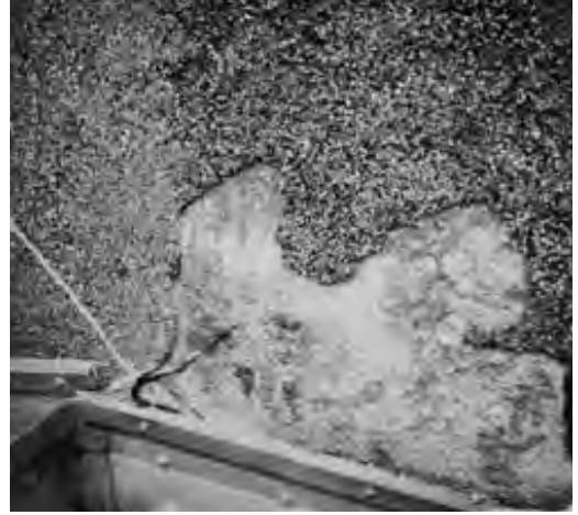
Figure 9.7. Expansion cracking caused the shotcrete surfaces to delaminate. Conservation of the deteriorated shotcrete is being planned.
