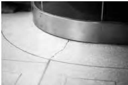
Figure 30.5. Differential settlement in the entrance of this Washington, D.C., apartment building has caused the terrazzo to crack. The durability of most terrazzo installations is largely a function of the structural stability of the system supporting the terrazzo.
