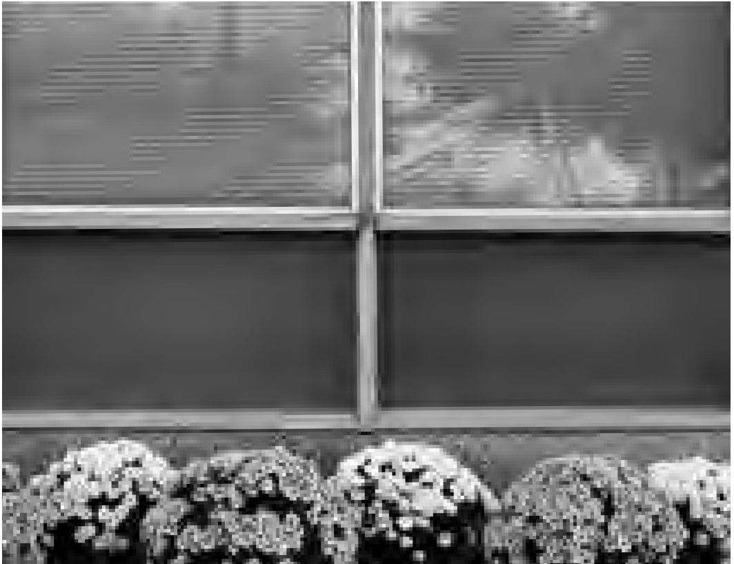
Figure 26.5. Finding spandrel glass to match historic colors is difficult. When an inappropriate replacement is installed (as in the left lower panel), the visual flaws are immediately apparent and compromise the building's character.
