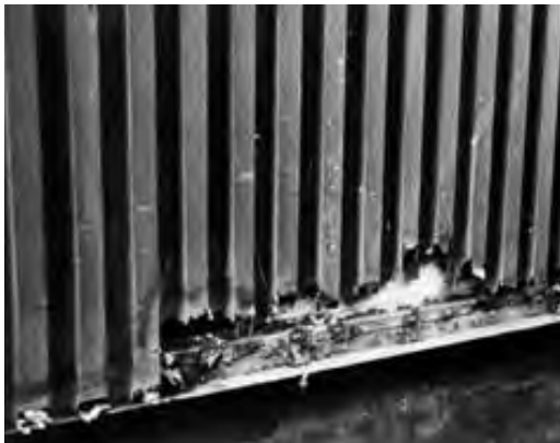
Figure 5.3. Corrosion of weathering steel is accelerated when water pools on surfaces, joints, and crevices.
