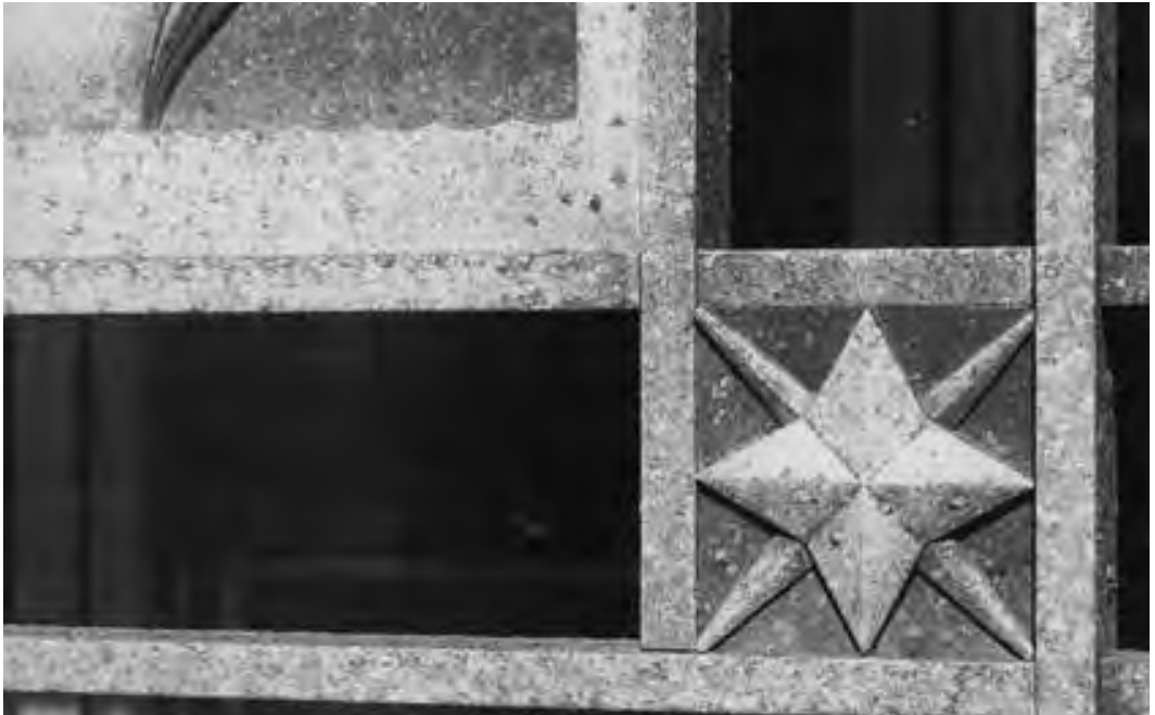
Figure 4.7. When exposed to a highly polluted atmosphere, stainless steels will corrode and are then often mistaken for aluminum. The gates at the Federal Trade Commission (1937, Bennett, Parsons, and Frost), Washington, D.C., have pitted because dirt on the surface has trapped moisture and created local electrolytic cells. Stainless steel should be cleaned periodically with water and a mild detergent.
