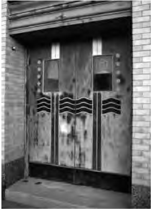
Figure 13.4. Decorative plastic laminates on the doors of the old Schine's Theater (1935, John Eberson), Auburn, N.Y., have faded from exposure to sunlight and have abraded from use.
