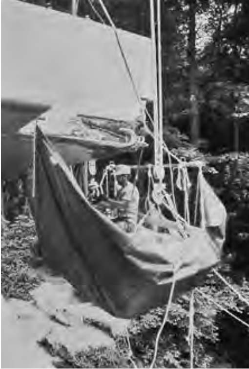
Figure 8.7. At Fallingwater (1937, Frank Lloyd Wright), Mill Run, Pa., conservators in suspended scaffolding assess deterioration of reinforced concrete.
