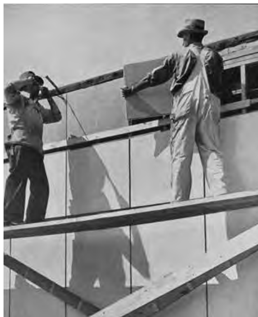
Figure 33.3. Porcelain enamel panels are installed sequentially to a wood-framed structure in the late 1930s. The panels were fastened by hand.
