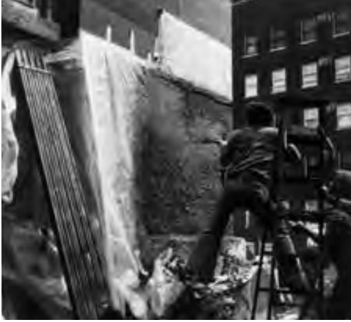
Figure 9.6. Wet-mix shotcrete, using pea-gravel aggregate from the original source, was applied to Unity Temple to match the original cast-in-place finish.
