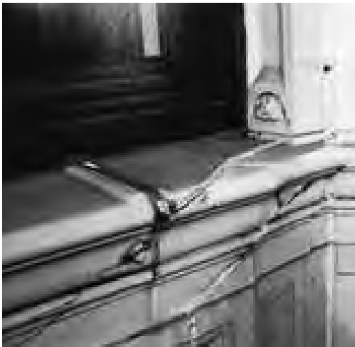
Figure 18.5. Terra cotta distress is often related to expansion corrosion of embedded metal anchorage elements.
