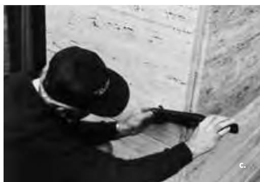
Figure 20.4a–c. The John F. Kennedy Center for the Performing Arts (1964, Edward Durell Stone), Washington, D.C. a. This was one of the first prominent buildings to be clad in thin stone veneer. b. Spalls, such as this one in a travertine panel, often occur at concealed metal anchors. c. Torque testing of a remedial expansion anchor installed in a precast concrete backup ensures that the panel is properly attached.
