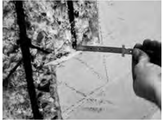
Figure 8.8. Cracking (top) can be caused by freeze-thaw cycles.
