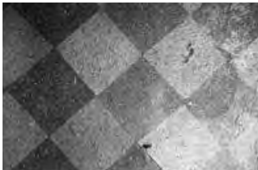
Figure 27.8. This worn linoleum shows the effects of abrasion and indentations. Some edges are beginning to lift up, usually a sign of water damage.
