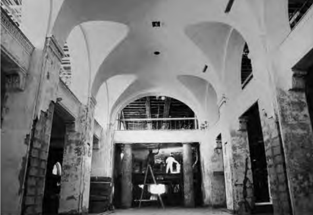
Figure 19.6 During restoration of the Vinoy Park Hotel (1925, Henry L. Taylor), St. Petersburg, Fla., deteriorated gypsum furring tiles in the lobby were replaced with concrete blocks, visible in the columns.
