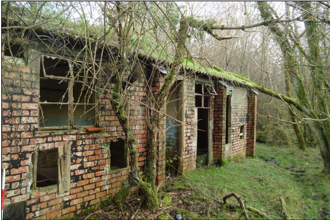
Plate 10: West facing elevation of the drying room and latrine block. Note the square holes added beneath the windows to fill the troughs inside
