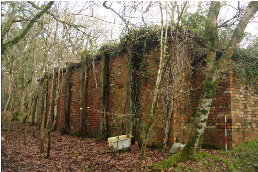
Plate 14: West facing elevation of the Hardened Sleeping Shelter. Note the reinforced banding
