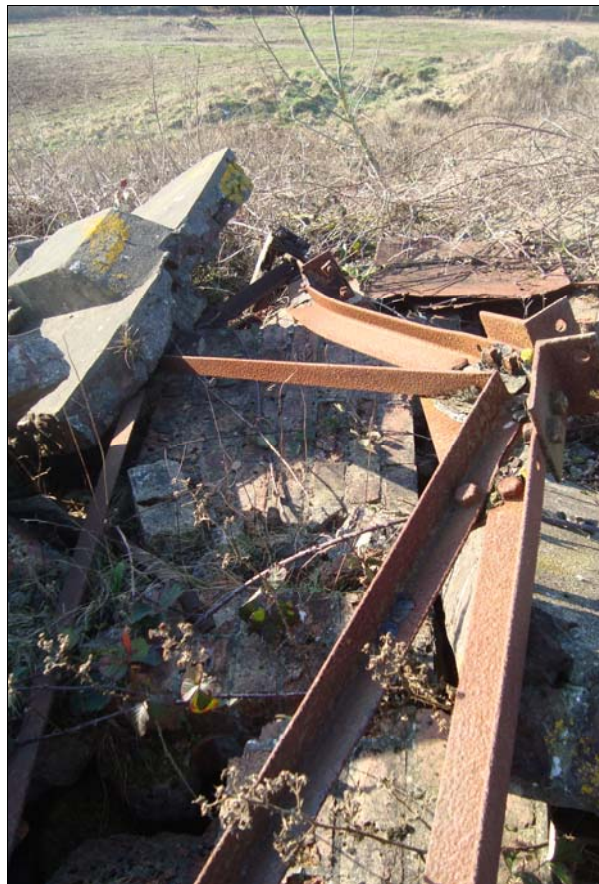
Plate 51: Remains of the roof trusses and external wall
