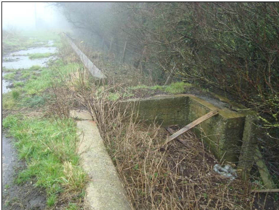
Plate 69: Remains of the side entrance to the Robin hangar. View to the north
