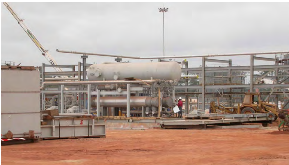
Plate A.2.1: Part of the oil heating apparatus at Pump Station 3 (Bélabo)
