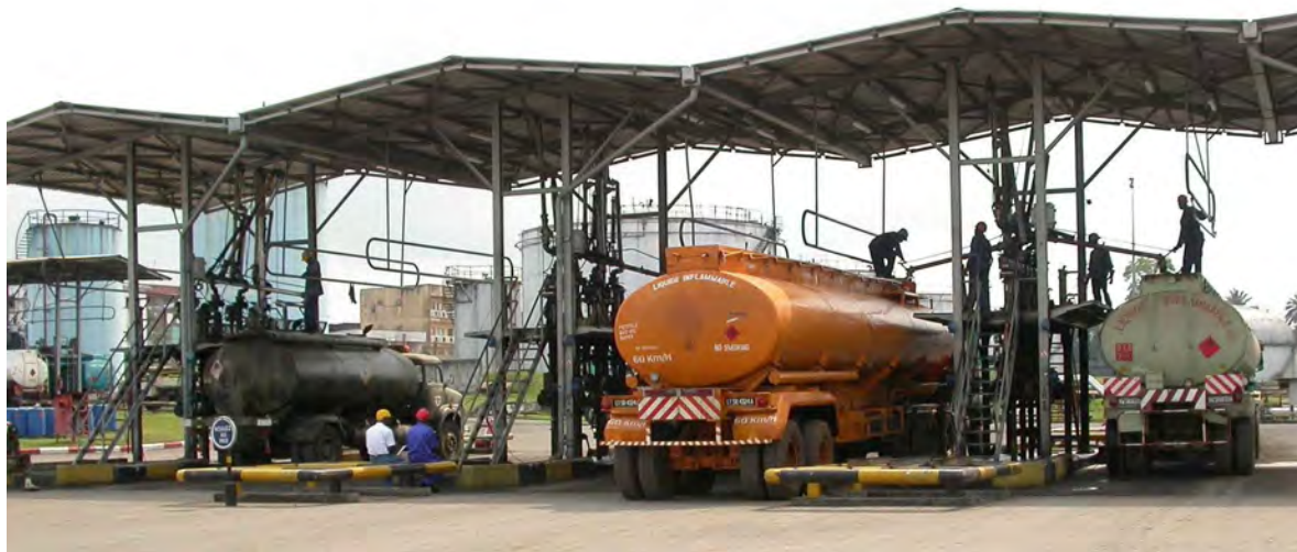
Plate A.2.3: Loading and offloading gantry at SCDP storage depot in Douala
