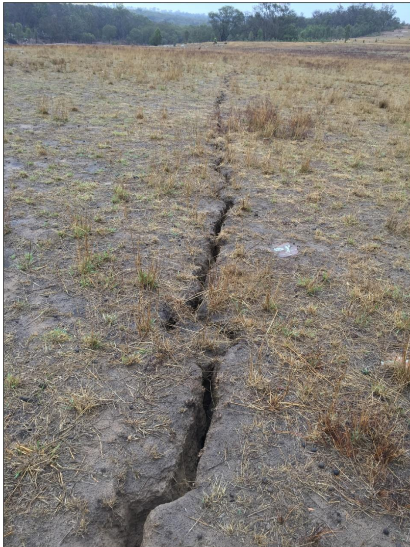
Figure 6: Surface crack that crosses H Line.
