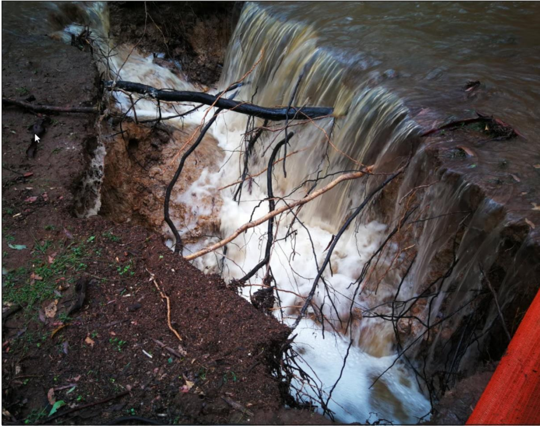
a) Example of flow into a subsidence crack during an overland flow event.
