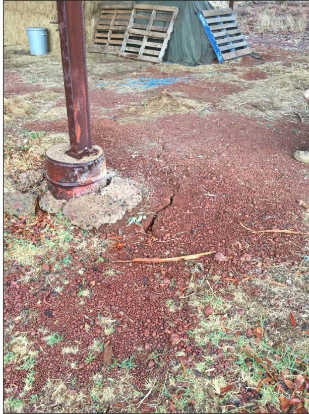
a) Cracking near foundation.
