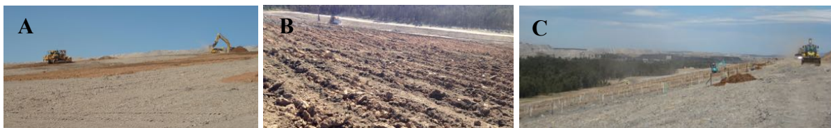
Plate 3.2. Setting up the experimental site. A) Subsoil (orange) and OGM (brown) have been layered over the spoil (grey). Piles of mulch are visible at the top of the site waiting to be spread after several ripping passes shown in B). In C) The plots have been set up and some additional mulch is being spread by the small excavator which also fixed the drains which had been put in previously with a dozer.
